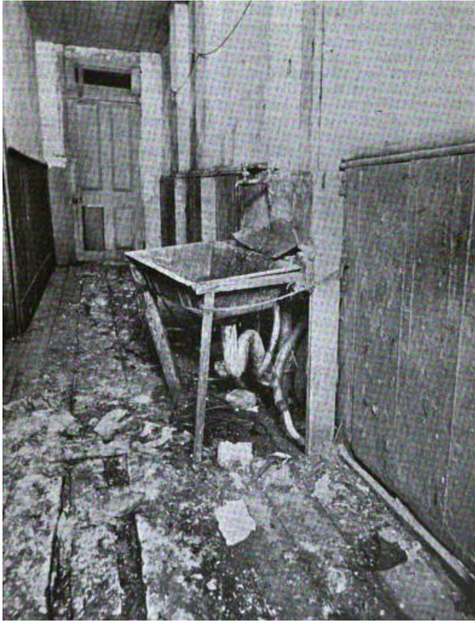
Photo 1.7: Public hall and sink. Sink supported only by string and flimsy wooden props. Hall floor covered with fecal matter and sewage. (1903)
