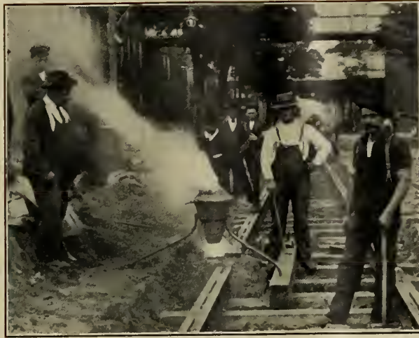
WELDING TROLLEY RAIL AT HOLYOKE, MASS.
