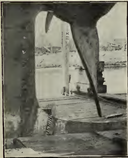
Fracture in Sternpost of U. S. S. "Gen. Nathaniel Greene," Opened Up by Drilling Preliminary to Welding.
