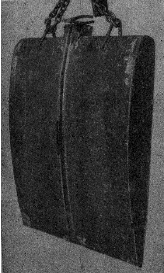
Fig. 12. Odd-shaped article welded by the electric slag process with a consumable electrode guide
