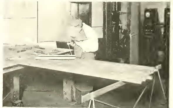
Fig. 95 Welding door hangers for fireproof steel doors. The square tubes on the horse are also arc welded on the seams.
