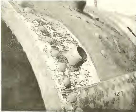
Fig. 66. Welder repairs to bottom blow-off valve of vertical boiler. The corroded plate was made good, the leaky rivet heads were welded over with new metal, and a new blow-off valve socket welded in. This repair saved replacing 50 sq. ft. of boiler plate, or scrapping the entire boiler.
