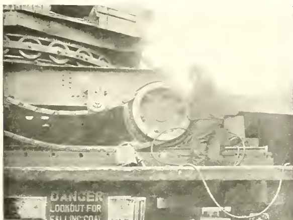
Fig. 63. Welding a coal shovel in the Great Lakes district. Arc Welding can be done at any point where an electric cable can be carried.
