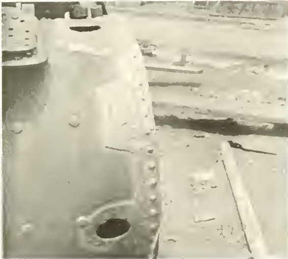
Fig. 101. Hoisting Engine Boiler, in which a large part of the flange had been badly corroded by use of poor water. This damage was completely repaired by a Lincoln Arc Welder, saving the boiler which would otherwise have been scrapped.
