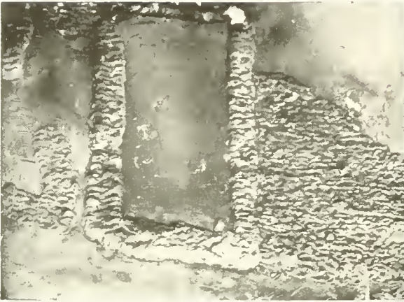
Fig. 100. Welded patch on steel kettle. The patch is clearly shown and also several portions around the patch which were built up by arc welding.
