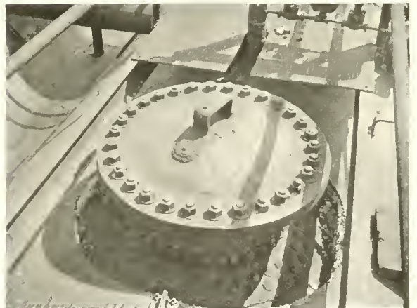
Fig. 71. Top of oil still showing welding, which makes these stills vapor tight. The Standard Oil Co. use the Lincoln Arc Welder on all their stills.
