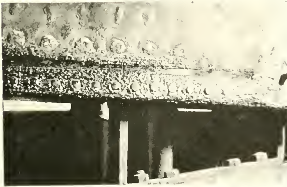
Fig. 45. A patch built up around a locomotive mud ring. This patch is nearly 8 feet long and made a saving in cost of over $2,000, besides the saving of a month's delay in making the repair.
