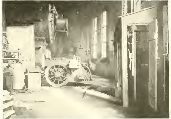
Fig. 52. Lincoln Arc Welder (Stationary Type) installed in engine house on large railroad.
