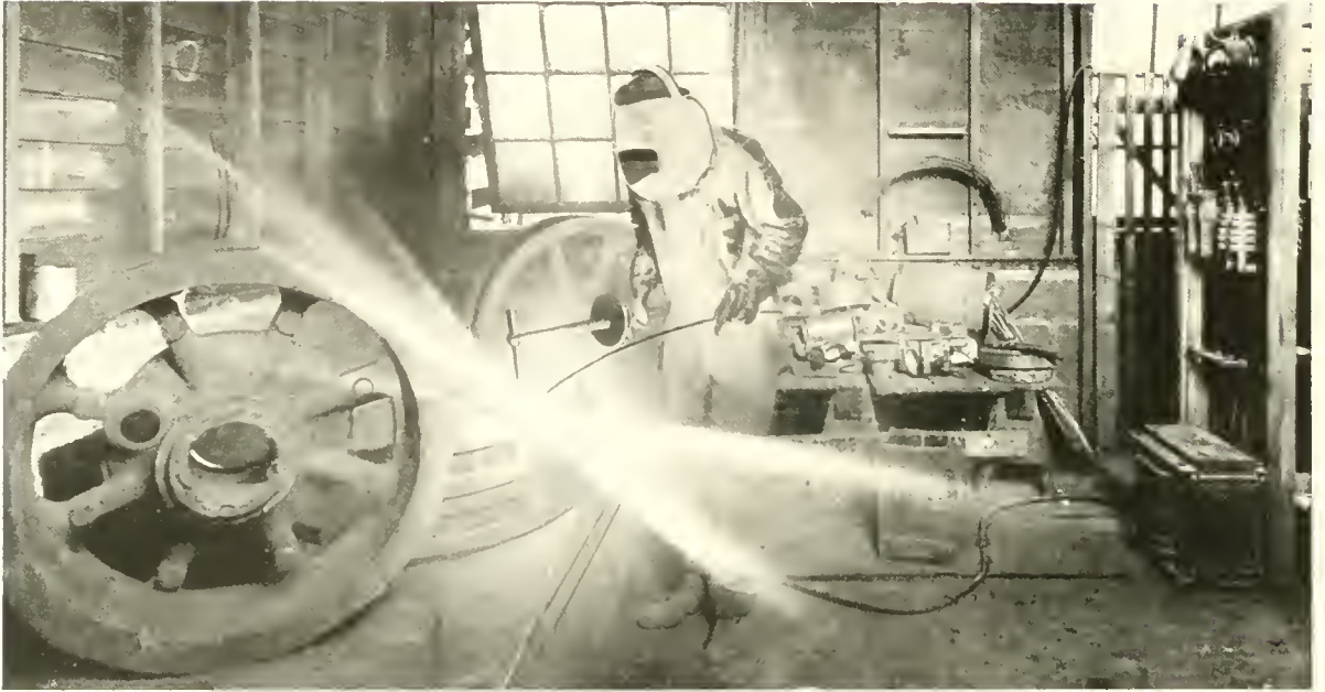
Fig. 16. Filling blow hole in a cast steel motor truck wheel. These castings, though subject to severe strain, were approved for use in military motor trucks when defects were repaired with the electric arc.
