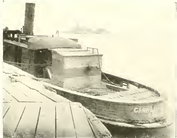
Fig. 60. Repair Tug, Carrie A. Ryerson , property of A. J. Mitchell & Son, Chicago. This tug carries a 200 ampere Lincoln Arc Welding outfit in the small house on the deck. This Welder is driven by a Novo Gasoline Engine and by actual test it performed the same amount of work on 6 gallons of gasoline as a constant voltage type of welder owned by the same company, driven by a steam turbine and consuming 7 tons of coal. (See page 48 for description of Constant and Variable Voltage Welders.)
