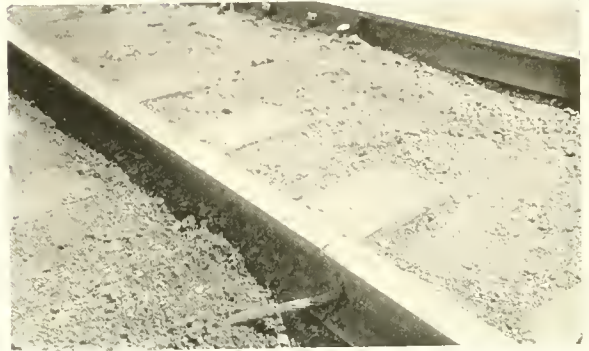
Fig. 4. A rail which has been welded together by the oxy-acetylene process but owing to the severe contraction of the metal on cooling the rail has broken.
