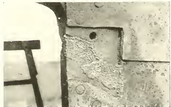
Fig. 62. Stern post on S. S. Cygnus (See Fig. 61). The weld was made with a Lincoln Arc Welder and was practically completed when this photograph was taken.
