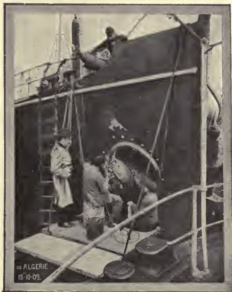
Fig. 211.—Repair of a hawse-hole of a steamship. In order to avoid wear by friction a welding rod without silicon is employed so as to obtain a hard metal.
