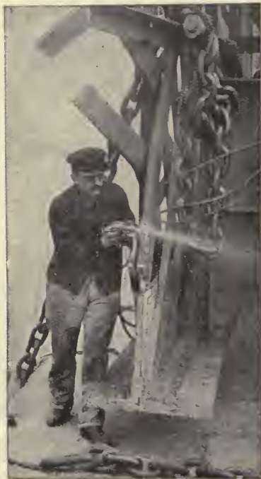
Fig. 256.—Rapid demolition with the cutting blowpipe of a bridge which had collapsed and was obstructing the harbour at Havre.
