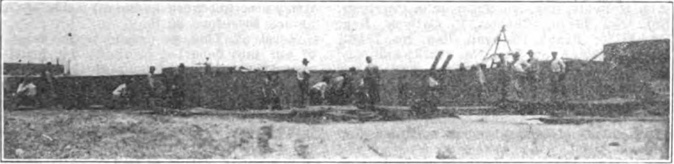
LOWERING BOTTOM 55,000 BARREL TANK, UNITED IRON WORKS JOB, UNION JOB, CUSHING, OKLA.
