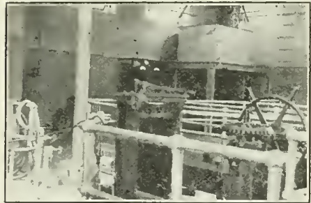
INTERIOR VIEW OF DYCKMAN STREET SEWAGE SCREENING PLANT, NEW YORK CITY.
