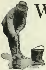
The hole to be patched is cleaned and the bottom and sides are painted with "Tarvia-KP."
