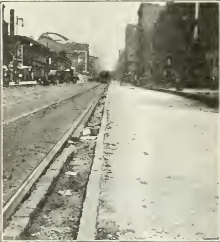
PAVEMENT RECONSTRUCTION ON WABASH AVE., CHICAGO, SHOWING GRANITE HEADER AND NEW PORTLAND CEMENT CONCRETE BASE IN PLACE, STREET CAR RAILS AND PAVING NOT DISTURBED.
