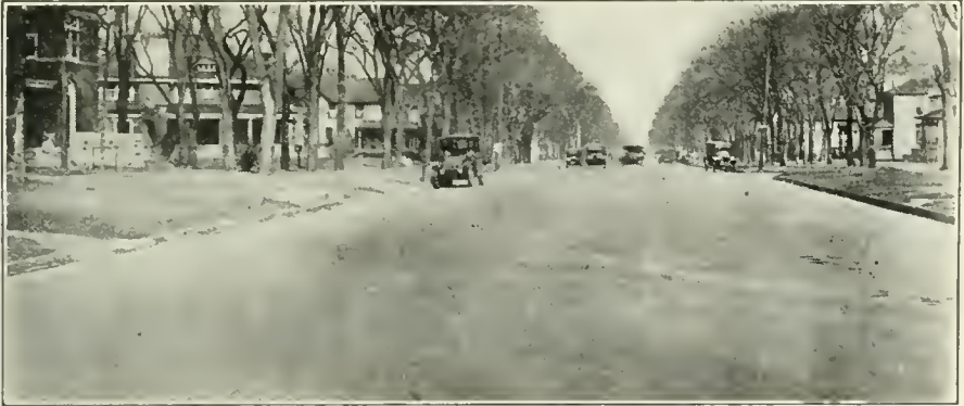
A WORN-OUT PAVEMENT ON TOPEKA AVE., TOPEKA, KANS., AFTER FULL RESURFACING WITH TEXACO ASPHALTIC CONCRETE. Street Resurfaced in 1917, Photograph Taken Jan. 11, 1921.
