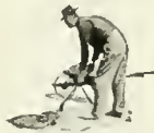
The mixture of "Tarvia-KP," stone and sand, is placed in the prepared hole.
