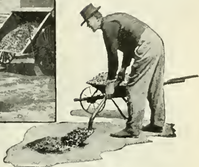
The mixture of "Tarvia-KP," stone and sand is put in the prepared hole.
