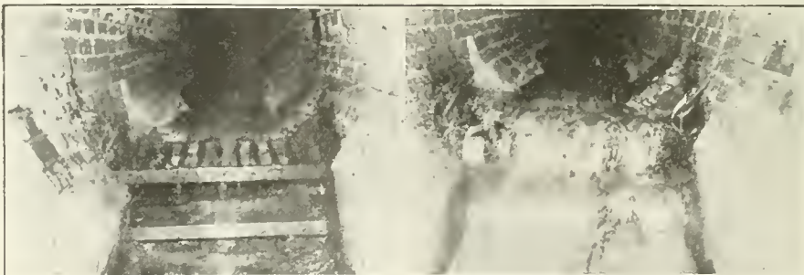
FIG. 4.—VIEW OF LEAPING WEIR. DRY WEATHER FLOW DROPS THROUGH THIS GRATING WHILE LARGE AMOUNTS OF RAIN WATER PASS OVER IT AND FLOW DOWN THE SEWER. FIG. 5.—THE GRATING CLOGS SOMETIMES WITH LEAVES, STICKS, RAGS, PAPER, ETC., WASHED INTO THE SEWER.
