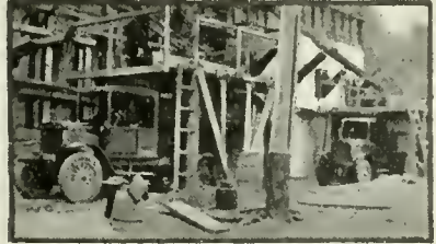
Sand and gravel bins with measuring boxes under which trucks drive for loading in less than 15 seconds.
