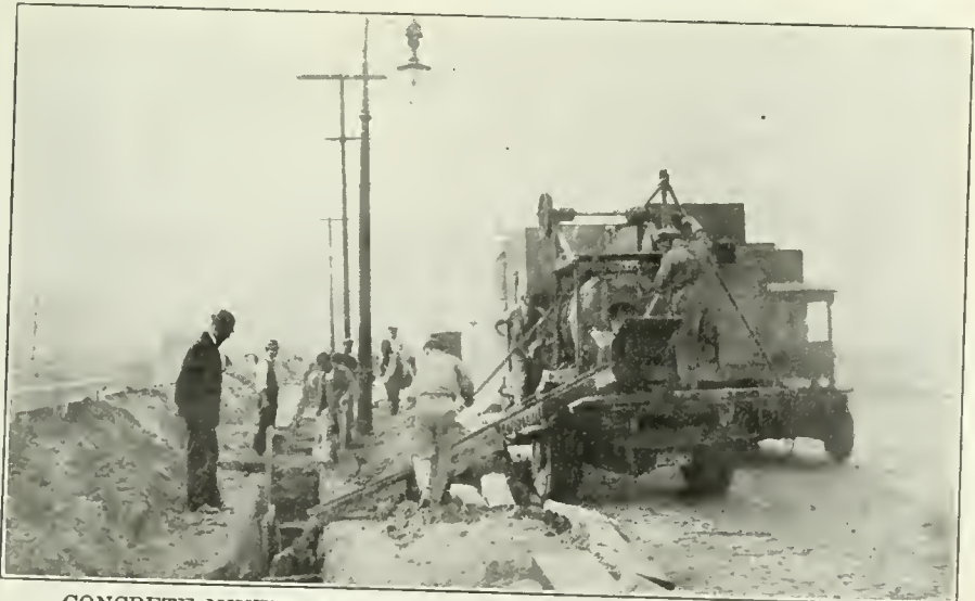
CONCRETE MIXER, TWO GRAVITY AGGREGATE HOPPERS AND WATER TANK, MOUNTED ON 7-TON PACKARD TRUCK FOR CONCRETING TELEPHONE CONDUIT IN NEW JERSEY.
