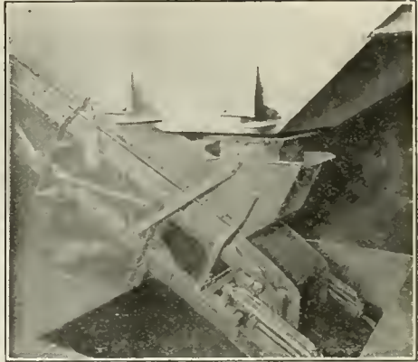
FIG. 3—CONVEYOR BENEATH TRACK HOPPER.
