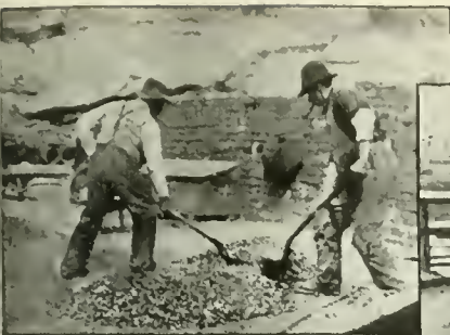
"Tarvia-KP" and stone are turned over by hand until all stones are coated. Then sand is added.
