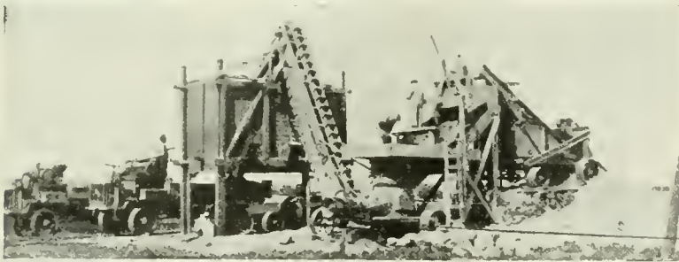
ARRANGEMENT OF EXCAVATOR AND PORTABLE ROCK CRUSHER AT GREEN LAKE COUNTY GRAVEL PLANT AT MANCHESTER, WIS.
