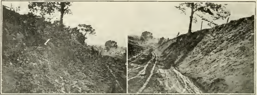
VIEWS SHOWING USE OF EXPLOSIVES FOR SLOPING ROAD BANKS. Left: Left Bank Immediately After Blasting. Right: Slope Complete on Right Bank.
