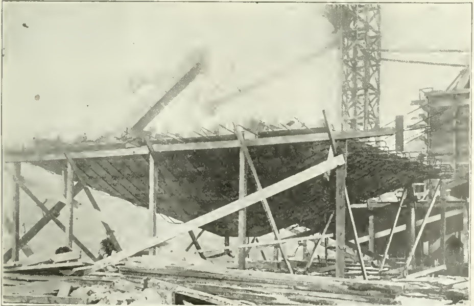
FIG. 5. RACKS FOR SUPPORTING STEEL IN IMHOFF TANK CONSTRUCTION, WESTERY SEWAGE TREATMENT WORKS, CLEVELAND, OHIO.
