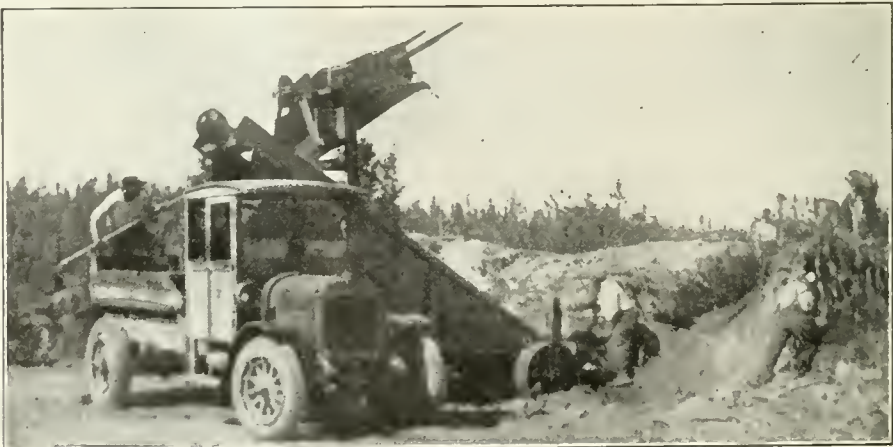
SMITH EXCAVATOR AND LOADER WORKING AT GRAVEL PIT FOR ST. LOUIS COUNTY, MINN.
