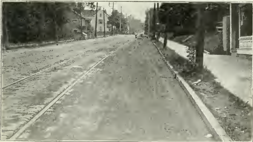
CARTHAGE PIKE, ST. BERNARD, OHIO, SHOWING NEW GRANITE PAVEMENT WITH GRANITE HEADER AND TEXACO ASPHALT FILLER, WITH OLD CAR TRACK PAVING LEFT UNDISTURBED.
