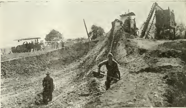
ABOUT 10,000 CU. YDS. OF GRAVEL HAVE BEEN REMOVED FROM THIS MANCHESTER, WIS., PIT WITHOUT MOVING THE EXCAVATOR.
