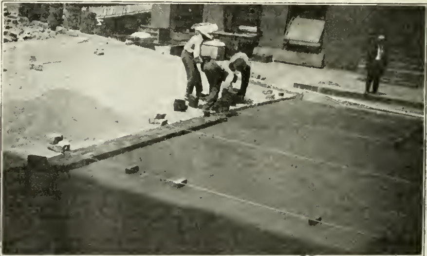
(Photograph by Courtesy The Barrett Co.) LAYING WOOD BLOCK PAVEMENT OVER TAR-SAND CUSHION ON EAST WATER ST., SYRACUSE, N. Y.
