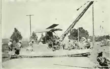
CONSTRUCTING "SECOND STORY" WORK ON STATE HIGHWAY IN LOS ANGELES COUNTY, CALIF.
