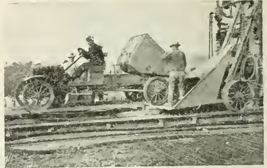
LIGHT TRUCKS WITH LEE BODIES DUMP AGGREGATE DIRECTLY INTO MIXER SKIP. WHEN PAVER MOVES TURN-TABLE IS MOVED WITH A TRUCK.
