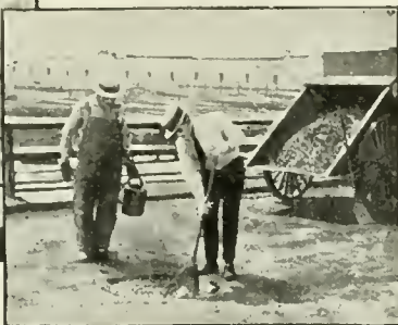
The hole to be patched is cleaned out and the bottom and sides are painted with "Tarvia-KP."
