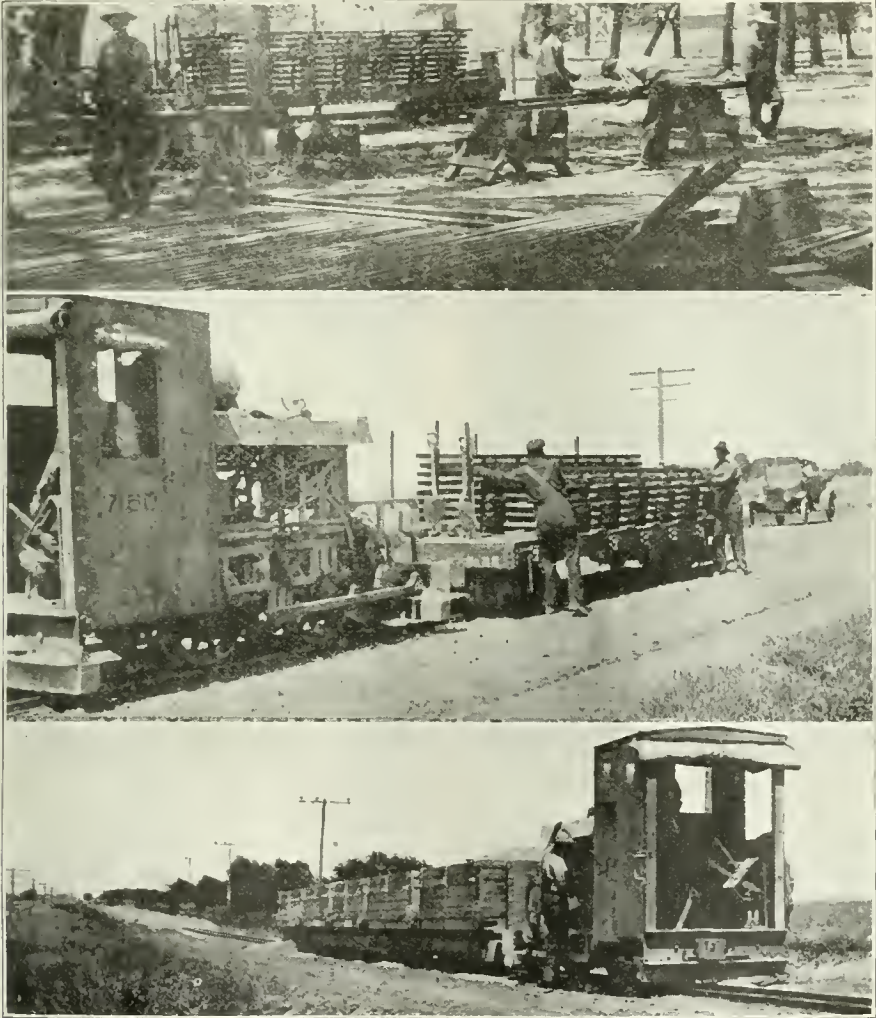
USING INDUSTRIAL RAILWAY ON GRAVEL ROAD CONSTRUCTION IN NEBRASKA. Top: Stock Pile of Rails, Horses on Which Sections of Track Are Assembled, and Car of Assembled Sections Ready to Go Out on Road. Center: Car of Assembled Sections of Track at End of Line Ready to Be Laid. Bottom: Gravel Dumped on Road and Train Used for Hauling It.
