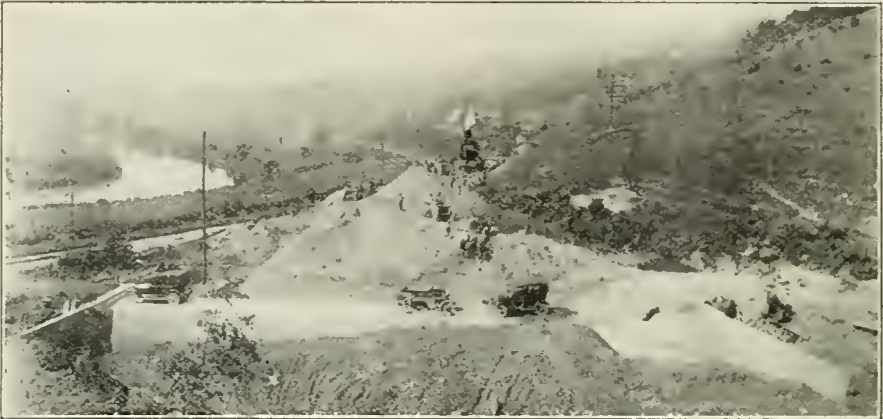
ONE OF THREE STEAM SHOVELS EXCAVATING MATERIAL FOR A 40-FT. FILL 250 FT. LONG, ON McMULLEN (MD.) HIGHWAY.
