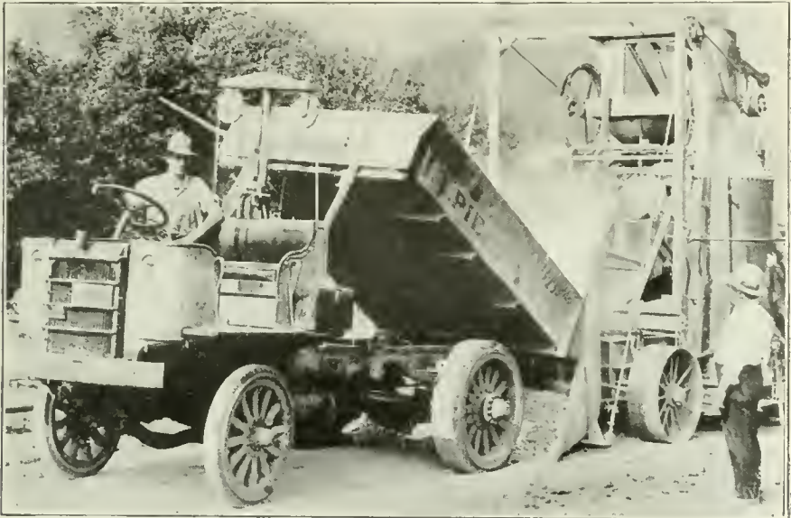
GARFORD 3\frac{1}{2} -TON TRUCK WITH PARTITIONED BODY DUMPING CONCRET- ING MATERIAL DIRECT TO MIXER LOADING SKIP.
