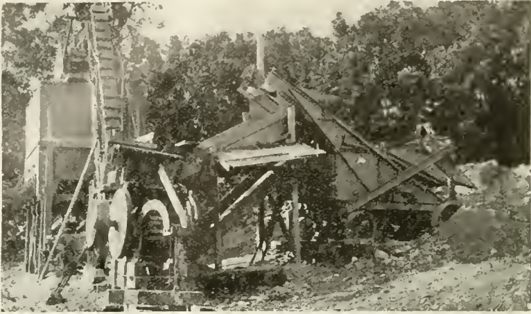
ARRANGEMENT OF GRAVEL PLANT AT DALTON, WIS.
