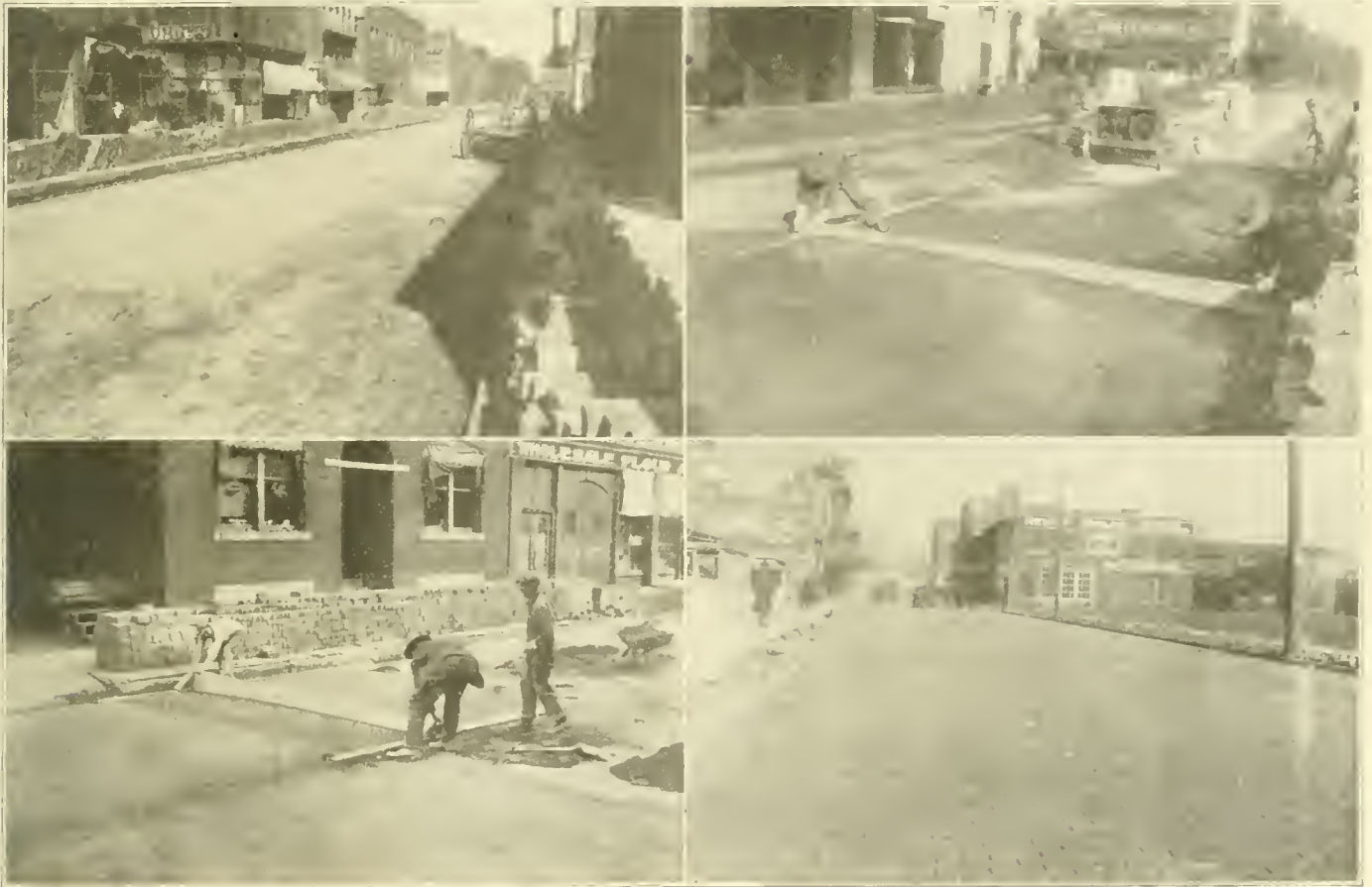
CONSTRUCTING NEW BRICK SURFACE ON OLD BRICK PAVEMENT ON WASHINGTON AVE., DANVILLE, ILL. Top Row—Left: Old Lower Course Brick Ready for Concrete. Right: Spreading a Smoothing Layer of Concrete Over Old Base. Lower Row: Spreading Sand Cushion—The New Surface Before Filling.
