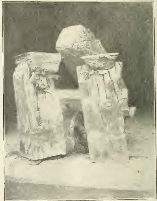
FIG. 2. VIEW OF DECAYED POSTS REMOVED FROM A MINNEAPOLIS BUILDING.
