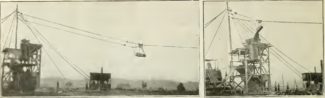
FIG. 3.—VIEWS OF SMALL SIZE EQUIPMENT INSTALLED BY ROAD COMMISSIONERS OF A MICHIGAN TOWNSHIP. THIS PLANT PRODUCES SAND AND GRAVEL SUFFICIENT FOR ALL THE TOWNSHIP ROAD WORK.
