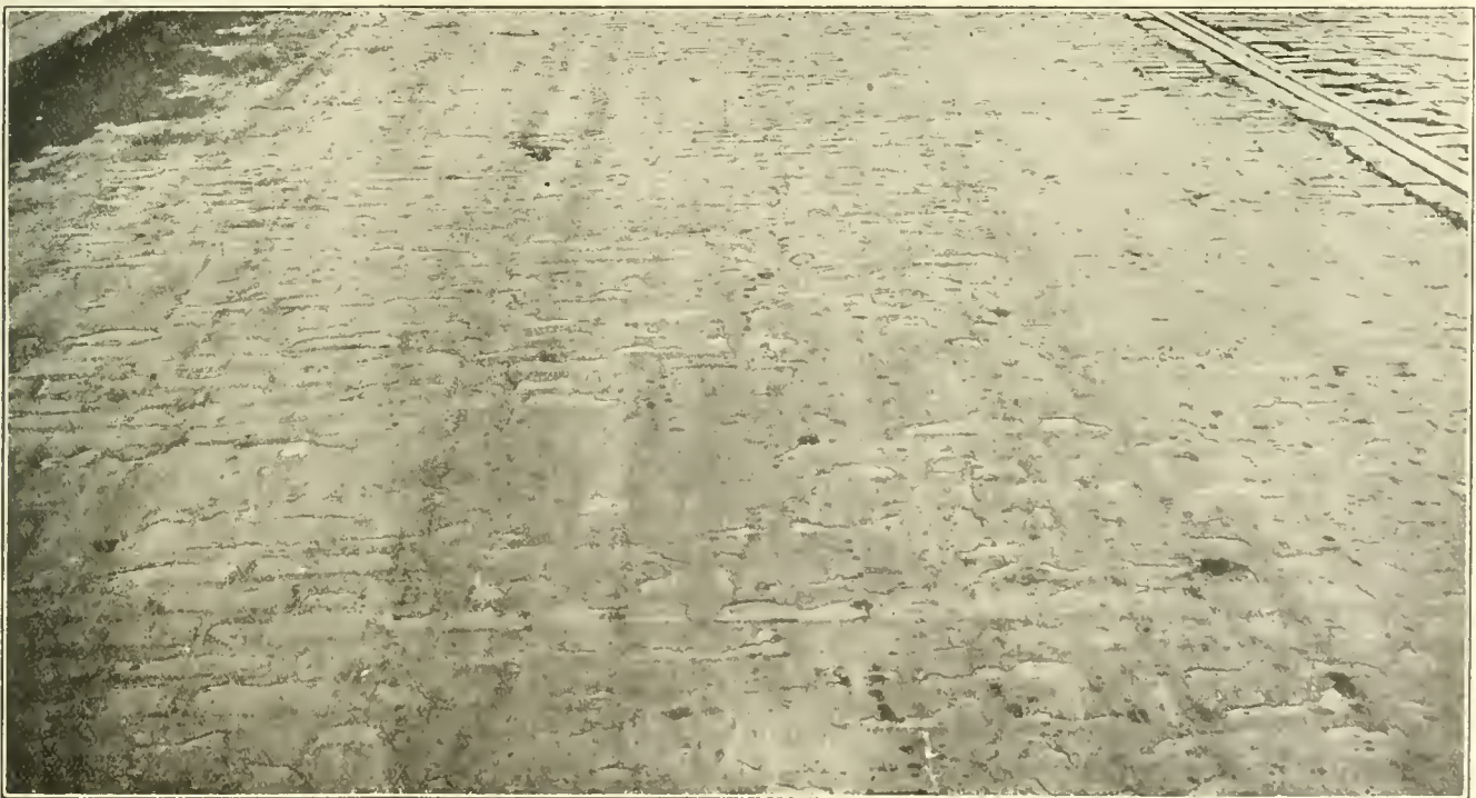
VIEW OF BRICK PAVEMENT, WITH ASPHALT FILLER, ON N. CRAWFORD AVE., CHICAGO, AFTER SEVEN YEARS OF SERVICE.
