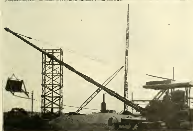
LADDER AND WHEEL TYPE EXCAVATORS AND BACKFILLER, OF PAWLING & HARNISCHFEGER MAKE, SHOWN IN OPERATION.
