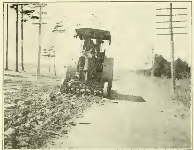
BREAKING UP SURFACE TREATED FOR A NUMBER OF YEARS WITH COLD REFINED TAR AT YORK, MAINE, WITH BUFFALO-PITTS SCARIFIER.
