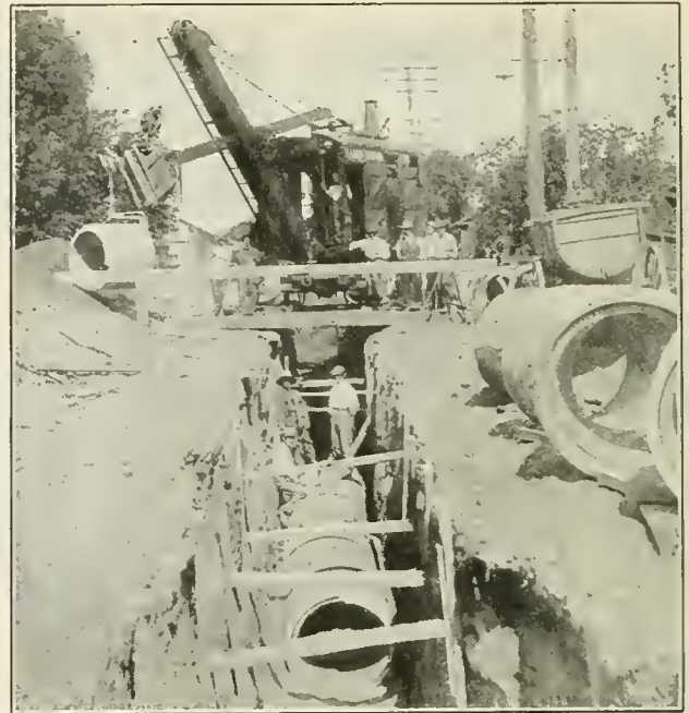
FIG. 2. THIS STEAM SHOVEL HAS DUG THE TRENCH, IS NOW LOWERING THE LARGE PIPE INTO PLACE AND WILL LATER BE USED FOR BACK-FILLING THE TRENCH.
