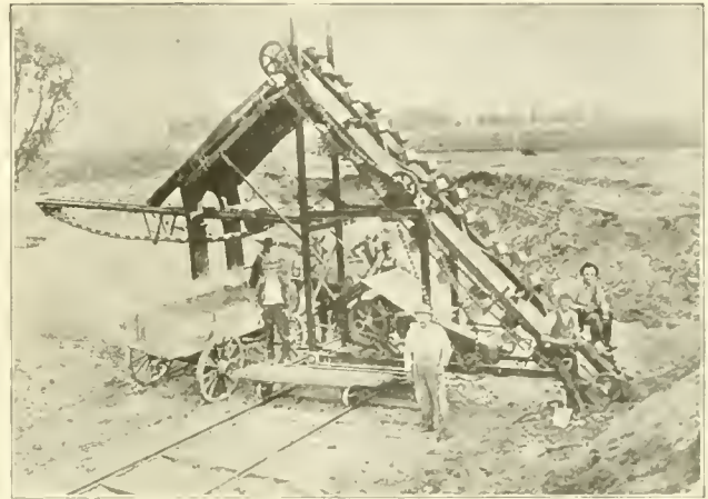
Calhoun County (Michigan) owns and operates four of these machines, and contractors own three others, making seven in the County.
