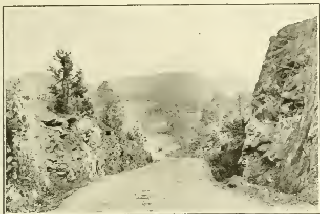
FIG. 1. ASHEVILLE-WILMINGTON-CHARLOTTE HIGHWAY, 18 FEET WIDE, CONSTRUCTED OF TEXACO ASPHALTIC CONCRETE OVER WORN-OUT MACADAM BASE.
