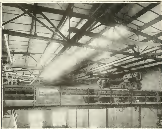
FIG. 1—THE LIGHT REFLECTING UNDER SURFACE OF GYPSUM TILE ON THE PHILADELPHIA SUBURBAN GAS CO. ROOF.
