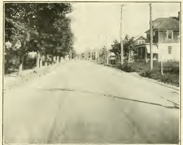
VIEW OF ASPHALT MACADAM HIGHWAY, BUILT BY PENETRATION METHOD, ON PUTNAM PIKE, TOWN OF JOHNSTON, RHODE ISLAND, AFTER THREE YEARS' SERVICE.
