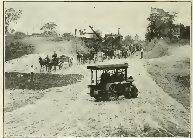
FIG. 1. REDUCING A GRADE WITH A MARION SHOVEL. The Wagons are Kept Loaded and the Shovel Sets the Pace for the Entire Outfit.
