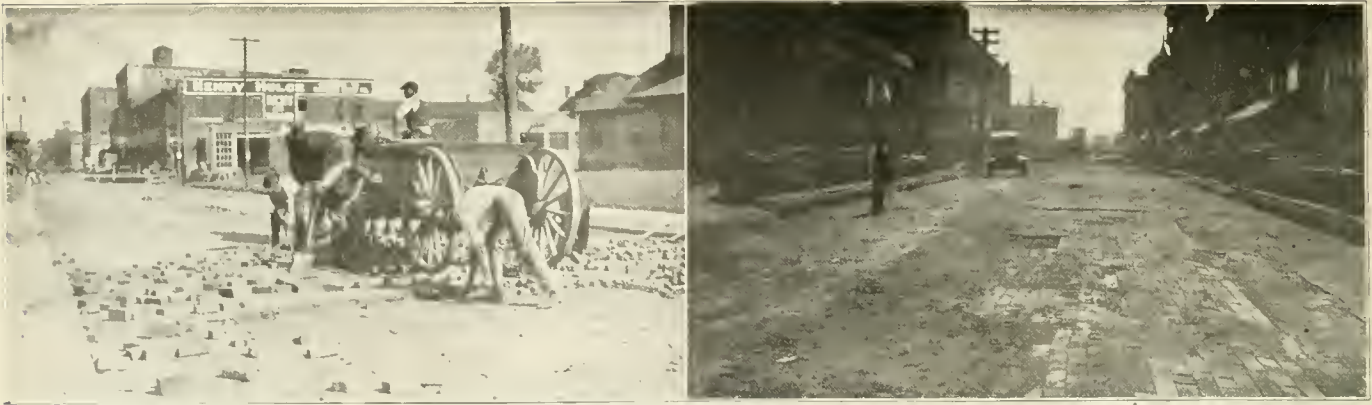
REMOVING TOP COURSE OF BRICK ON WASHINGTON AVE., DANVILLE, ILL.—BASE READY FOR CONCRETE ON SAME JOB.
