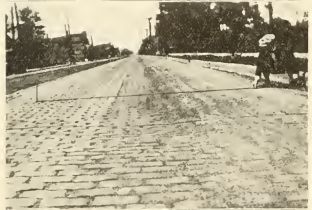
FAILURE OF 6-IN. CEMENT CONCRETE FOUNDATION TO ARCH OVER WEAK SUBGRADE. PAVEMENT CARRIES AVERAGE TRAFFIC INCLUDING A FAIR PERCENTAGE OF TRUCKS.
