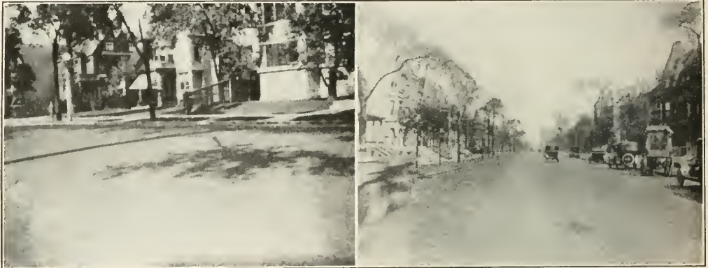
VIEWS OF WARRENITE-BITULITHIC PAVEMENT LAID OVER OLD MACADAM. Left: Sheridan Road, Chicago. Right: Michigan Boulevard, Chicago.
