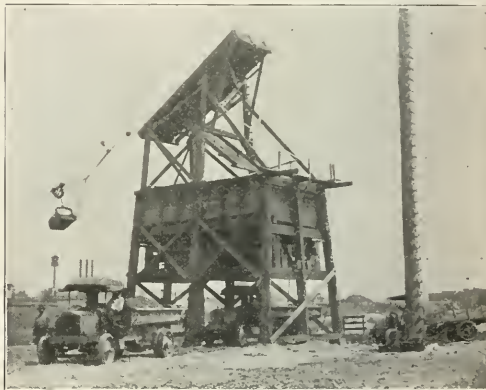
SAUERMAN DRAGLINE CABLEWAY EXCAVATOR CONVEYING GRAVEL TO BINS AT INDIANAPOLIS MUNICIPAL GRAVEL PLANT.
