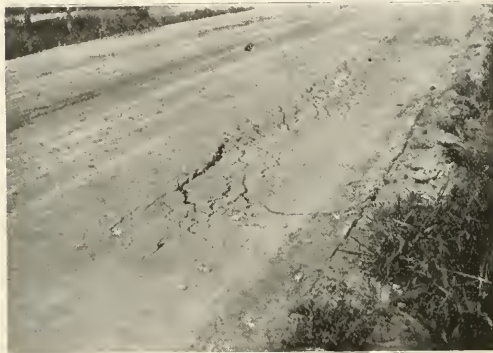
HEAVY TRAFFIC HIGHWAY RESURFACED WITH ASPHALTIC CONCRETE. FAILURE TO PROVIDE EDGING OR CURB PERMITTED LATERAL DISPLACEMENT WITH RESULT SHOWN. SUCH FAILURES NOT DUE TO TYPE OF PAVEMENT BUT TO POOR ENGINEERING.
