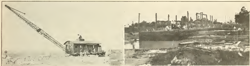
VIEWS OF CONSTRUCTION EQUIPMENT USED ON INTER-RIVER DRAINAGE DISTRICT. One of the Walking Dragline Excavators—Launching the Hull for One of the Floating Dredges.
