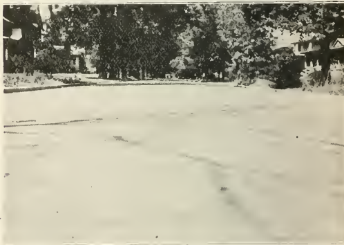
TWO-INCH ASPHALTIC CONCRETE LAID OVER OLD MACADAM 3½ YEARS AGO. OLD ROADBED CUT DOWN AT SIDES AND BUILT UP AT CROWN. PAVEMENT IN PERFECT CONDITION.
