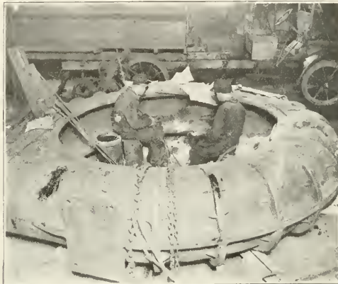
BUILDING UP WORN SURFACE OF "SAND SUCKER" DEPOSITING 1,264 LBS. OF HIGH CARBON STEEL WITH AID OF OXWELD OXY-ACETYLENE BLOWPIPES.
