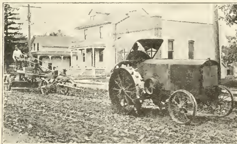
LAUSON TRACTOR DRAWING GRADER FOR CHEROKEE COUNTY HIGHWAY COMMISSION, GAFFNEY, S. C.
