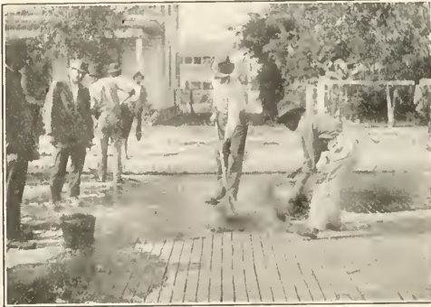
APPLICATION OF ASPHALTIC FILLER ON BRICK PAVEMENT BY THE SQUEEGEE METHOD, NEWPORT AVE., TAMPA, FLORIDA.
