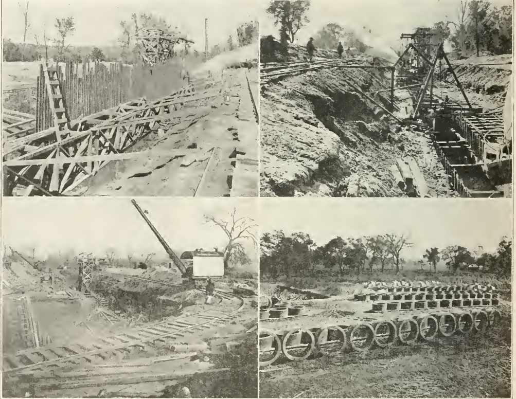
VIEWS ON THE CONSTRUCTION OF A WATER INFILTRATION GALLERY AT DES MOINES, IOWA.
