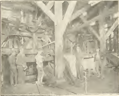
PLANT FOR GRINDING AND PULVERIZING KENTUCKY ROCK ASPHALT. EACH MACHINE HAS A CAPACITY OF 350 TONS PER 10 HOURS.
