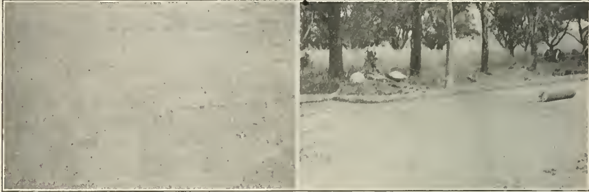
FIG. 3. THE BASE SHOWN IN FIG. 2 RESULTED IN AN UNEVEN FINISHED ASPHALT PAVEMENT. FIGS. 1, 2 AND 3 INDICATE HOW AN IMPROPERLY PREPARED SUBGRADE MAY PRODUCE IRREGULARITIES THROUGHOUT THE PAVEMENT STRUCTURE. FIG. 4. THE ROUGH IRREGULAR SURFACE OF AN IMPROPERLY FLOATED CONCRETE BASE.
