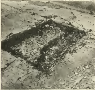
CRACK AND UPHEAVAL OF CEMENT CONCRETE FOUNDATION UNDER ASPHALTIC CONCRETE PAVEMENT, A COMMON RESULT OF THIS TYPE OF CONSTRUCTION.
