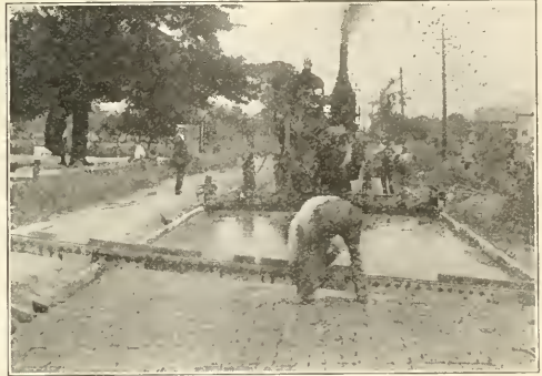
PARRISH AUTOMATIC CUTTING AND TAMPING TEMPLATE and FOOTE CONCRETE MIXER AT WORK ON ASHTABULA-CONNENAUT HIGHWAY, OHIO, MAIN ROAD FROM BUFFALO TO CLEVELAND. MONOLITHIC WIRE-CUT LUG BRICK CONSTRUCTION, STATE AND FEDERAL AID ROAD 12 MILES LONG.
