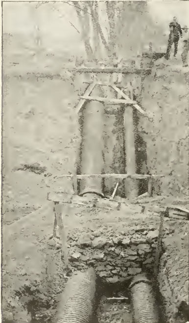
SIPHONS OF ARMC0 IRON CORRUGATED PIPE INSTALLED TO REPLACE WOODEN FLUME CARRYING IRRIGATION WATER ACROSS HIGHWAY.
