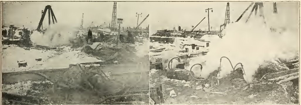
USING THE LIVE STEAM METHOD OF THAWING FROZEN GROUND BEFORE EXCAVATING FOR HOG ISLAND WATER AND SEWER LINES.
