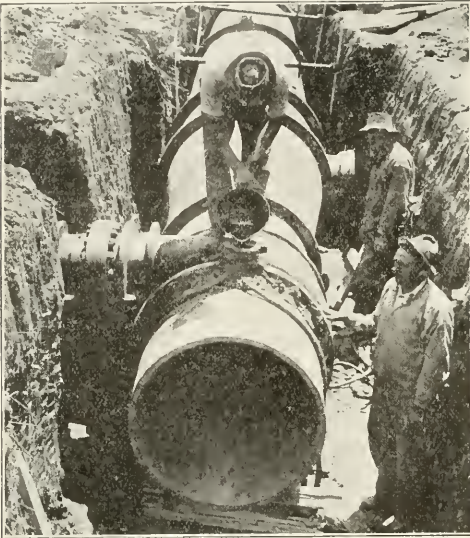
POURING METALIUM JOINTS. TESTS SINCE THE COMPLETION OF THIS 48-IN. MAIN INDICATE FREEDOM FROM LEAKAGE.
