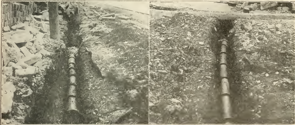
VIEWS SHOWING SPECIAL UNDERDRAINAGE OF NEW BRICK PAVEMENT ON WOODHILL ROAD IN CLEVELAND, OHIO.
