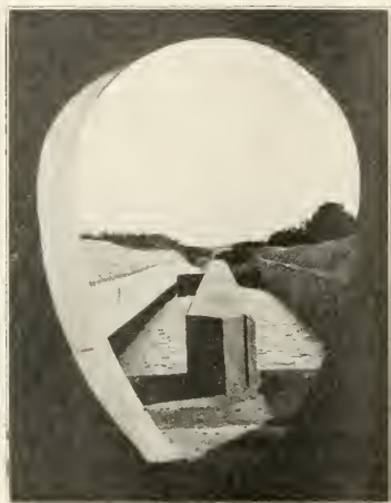
THE SEWAGE PASSES FROM SEWER THROUGH SETTLING TANK AND OPEN CHANNEL AT PAYSANDU TO RIVER BEYOND.
