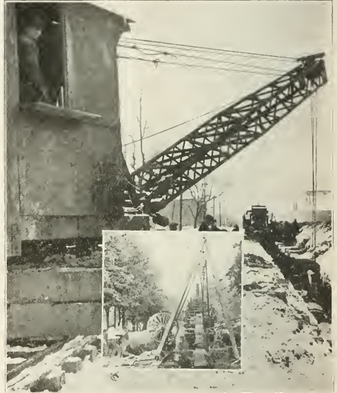
LOWERING 48-IN. PIPE INTO TRENCH. ONE MAN OPERATING CRANE AND ONE OR TWO HELPERS HANDLE ALL PIPE. INSERT SHOWS OLD METHOD WHEN SIX OR TEN MEN "RASSLED" WITH THE PIPE.
