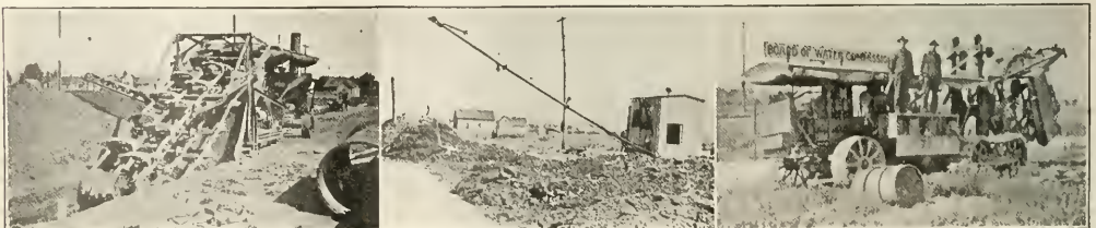
THREE OF THE MACHINES USED ON DETROIT WATER TRENCH CONSTRUCTION. AT LEFT IS AUSTIN TRENCHING MACHINE WORKING ON TRENCH 6 FT. WIDE AND 12 FT. DEEP. THE MIDDLE VIEW SHOWS AN AUSTIN BACKFILLER. THE VIEW AT RIGHT IS A BUCKEYE MACHINE USED ON DITCHING FOR 6 AND 8 IN. PIPE.
