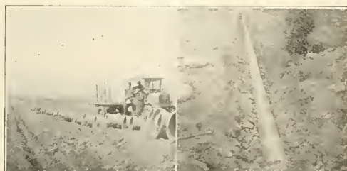
USING VITRIFIED CLAY PIPE IN IRRIGATION LINES. Motor Trucking the Pipe to the Trench—A Well Laid Line Ready for Backfilling.
