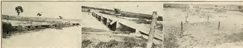
LOW WATER BRIDGES ON OKLAHOMA HIGHWAYS. Left: Upstream View of Concrete Low-Water Bridge after a Flood. Center: Downstream View of Same Bridge. Right: Wooden Floor and I-Beam Joists Were Carried Away by High Water.
