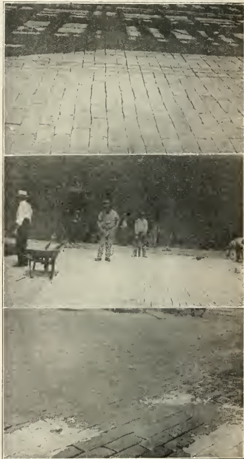
FIG. 4 (TOP): CORRECT METHOD OF LAYING STONE PAVING BLOCKS WITH THIN JOINTS. FIG. 5 (CENTER): BLOCKS RAMMED TO SOLID BEARING, TO EVEN CONTOUR AND TRUE CROSS-SECTION. FIG. 6 (BOTTOM): HOT MORTAR FLUSHED TO SURFACE OF BLOCKS AND PUSHED INTO JOINTS BY SQUEEGEES.
