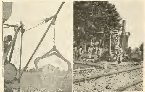
FIG. 3. BATCH TRANSFER ATTACHMENT FITTED WITH BAILETS TO LIFT BOXES FROM CARS. FIG. 6. FOUR MEN NEEDED AT DISCHARGE END OF MIXER.
