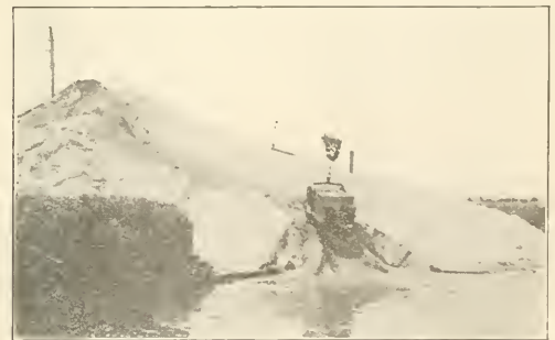
ONE OF LOGAN COUNTY (ILL.) GRAVEL PLANTS. Excavating Pit-run Material with Sauerman Dragline Cableway Excavator.
