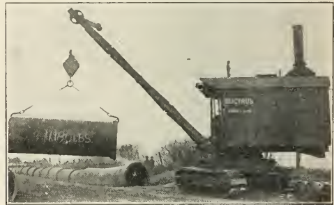
THIS IS HOW LARGE PIPE IS HANDLED. Bucyrus Steam Shovel-Cranes Replace Derricks for Stringing and Lowering Pipe.
