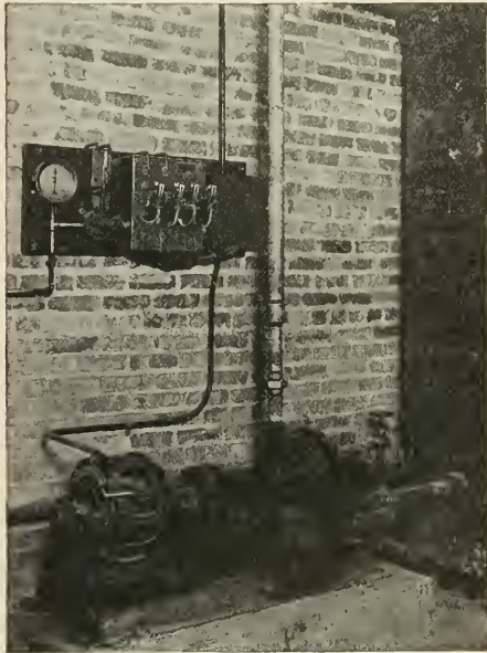
THREE H. P. 3-PHASE MOTOR DRIVING HOUSE PUMP CONTROLLED BY PRESSURE REGULATOR AND SELF-STARTER MOUNTED ON WALL.
