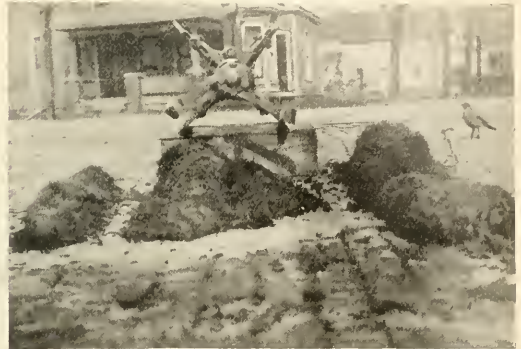
ROOTS REMOVED FROM GOSHEN, IND., SEWER WITH TURBINE SEWER CLEANER. ROOTS HAD COMPLETELY STOPPED FLOW AFTER TREES WERE CUT DOWN.
