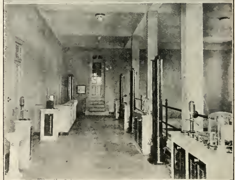
VIEWS OF PUMPING AND FILTERING EQUIPMENT OF WATER WORKS AT SALTO, URUGUAY.
