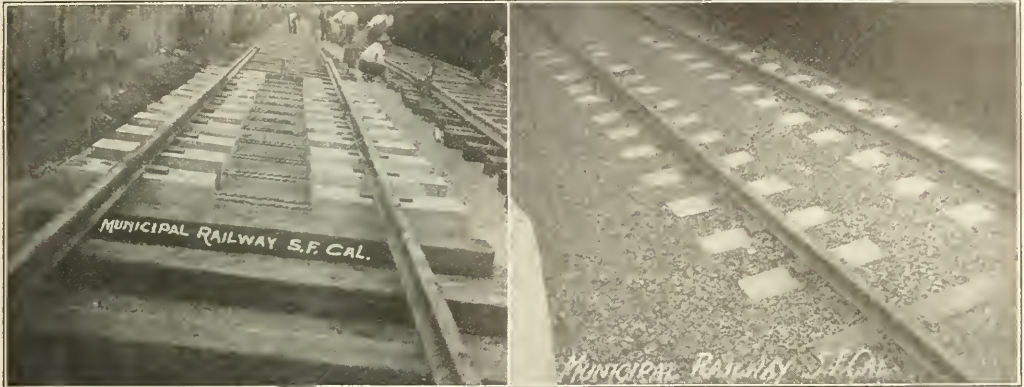
VIEWS OF OPEN CENTER REINFORCED CONCRETE TIES ON MUNICIPAL RAILWAY, SAN FRANCISCO. BEFORE AND AFTER PLACING BALLAST.
