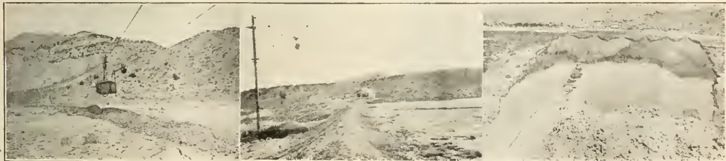
REMOVING SILT FROM IRRIGATION RESERVOIR WITH SAUERMAN ½ YD., LEVEE TYPE, DRAGLINE OUTFIT.
