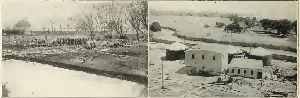
VIEWES OF THE DOMESTIC WATER FILTRATION PLANT AT HOG ISLAND, PA. Left: Foundations for Filter Tanks, East End. Right: View of Completed Plant.
