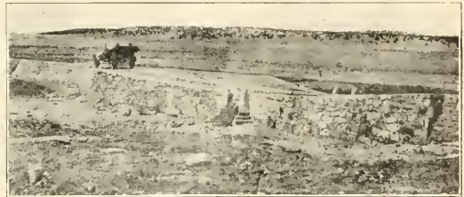
NO. 3—TYPE OF ROAD FLOORING USED IN NEW MEXICO WHERE ARROYO BED IS ROCK OR NOT LIKELY TO SCOUR BELOW FROM THE OVERFLOW.
