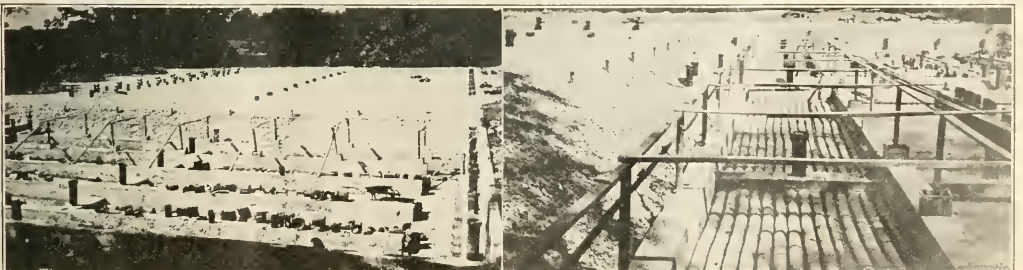
VIEWS OF SPRINKLING FILTER, SEDALIA, MO., SEWAGE TREATMENT PLANT.
