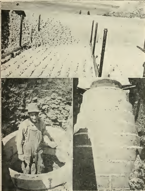
VIEWS OF SEWERAGE WORKS AT MT. HOREB, WIS. Top: Sprinkling Filter Under Construction. Bottom: Sewer Manhole of Cement Blocks Under Construction and Completed.
