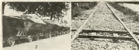
FIG. 7. CEMENT HAULED IN CARS FROM STORAGE SHEDS TO MIXER. FIG. 8. RIGID CROSSING MAKES DERAILMENT ALMOST IMPOSSIBLE.
