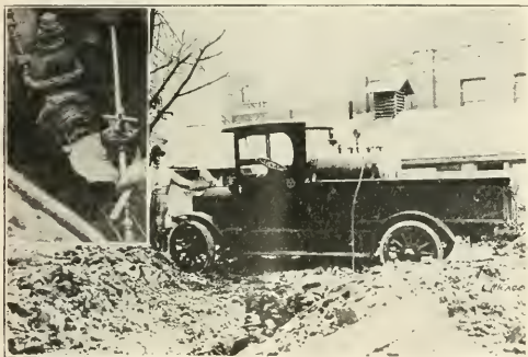
COMPRESSOR PLANT OF POWER TAPPING MACHINE MOUNTED ON 1½-TON G. M. C. MOTOR TRUCK. THE INSERT SHOWS THE TAPPING MACHINE IN THE TRENCH.
