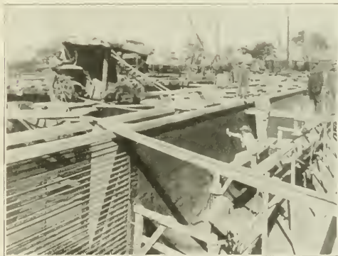
USING THE CEMENT GUN PROCESS TO CONSTRUCT 3-INCH WALLS IN COLUMBUS, OHIO, SEWAGE SETTLING TANKS.
