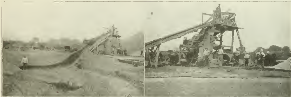
VIEWS OF PLANT FOR WASHING AND SCREENING DIRTY CINDERS FOR SEWAGE BEDS, ALLIANCE, OHIO. Dirty Cinders Hoisted Over Runway in Slip Scraper to Elevated Platform, Dumped into Screen, Washed While Screening, Discharged into Industrial Cars and Transported Back to Beds.
