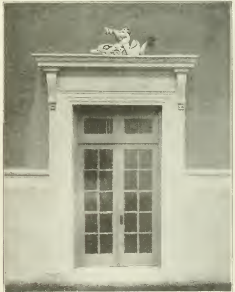
VIEW SHOWING DETAIL AROUND DOOR IN TOWER OF REINFORCED CONCRETE WATER TANK, MIAMI, FLA.—NOTE STUCCO FINISH.
