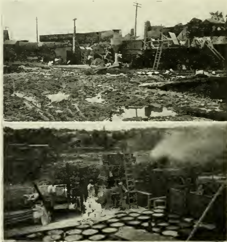
VIEWS OF ASPHALT MIXING PLANT OWNED AND OPERATED BY CITY OF WORCESTER, MASS.
