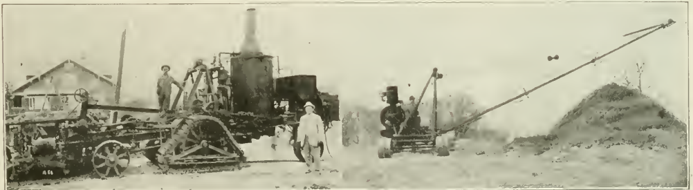
TYPES OF SEWER EXCAVATING AND BACKFILLING MACHINERY SUCCESSFULLY EMPLOYED BY CHICAGO CONTRACTORS.
