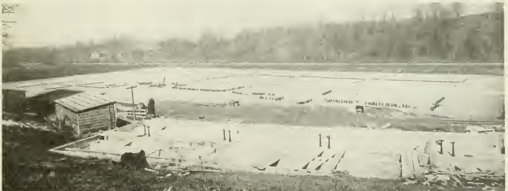
FIG. 5—VIEW OF NEW SEWAGE TREATMENT PLANT AT XENIA, OHIO.
