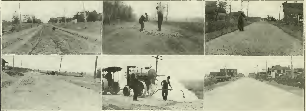
VIEWS ON THE CONSTRUCTION OF THE ASPHALTIC MACADAM DOLLAR BAY ROAD, HOUGHTON COUNTY, MICH.
