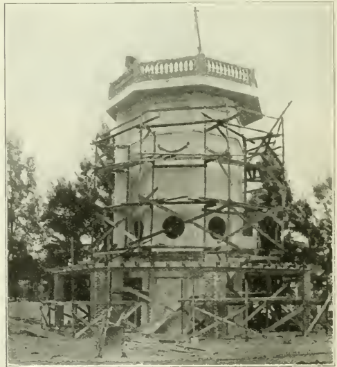
CONSTRUCTION VIEW OF EASTWOOD REINFORCED CONCRETE OBSERVATORY AND WATER TANK TOWER AT MIAMI, FLA.
