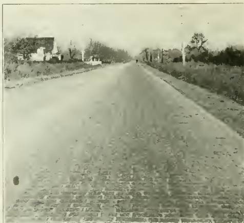
BRICK PAVEMENT, DANVILLE, ILL. WHERE CEMENT FILLER FAILED WIDTH OF PAVEMENT, BUT WIRE-CUT-LUG BRICK REMAINED PRACTICALLY PERFECT.
