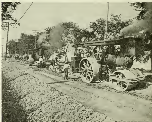
IN PREPARING THE GRADE FOR CONCRETE ROADS IN WAYNE COUNTY, MICH., MACHINERY IS USED WHENEVER POSSIBLE.
