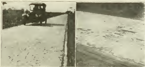
PAVEMENT FAILURE DUE TO CARELESS CONSTRUCTION.
