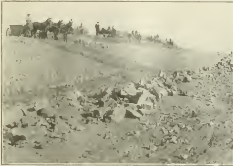
VIEW OF GRADING OUTFIT ON LEAN SPRINGS IRRIGATION RESERVOIR CONSTRUCTION IN TEXAS.
