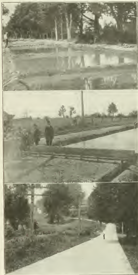
UPPER—CURING CONCRETE PAVEMENT BY PONDING, BELLEVUE AVE., HAMMONTON, N. J. MIDDLE—SETTING KAHN ARMOR PLATE IN PROPER POSITION BY USE OF INSTALLING DEVICE. LOWER—VIEW ON BALTIMORE PIKE, A 22-MILE CONCRETE ROAD, NEAR WAWA, PA.
