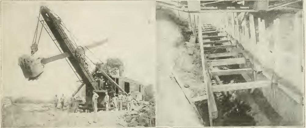
EXCAVATING FOR LARGE SEWERS IN CHICAGO WITH 70-TON MARION STEAM SHOVEL. Note Method of Supporting Shovel Over Trench on Truss and Rollers. Lower View Shows Trench in Sand Under Shovel.
