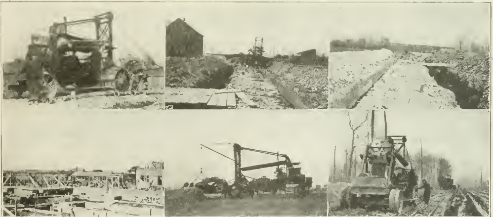
VIEWS OF P. & H. TRENCHING MACHINE IN SUCCESSFUL OPERATION UNDER ADVERSE CONDITIONS BY ERIE (PA.) WATER DEPARTMENT.
