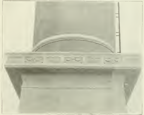
VIEW SHOWING DETAIL AROUND THE BALCONY OF THE REINFORCED CONCRETE WATER TANK ON CARL FISHER'S ESTATES, ALTON BEACH, MIAMI, FLA.
