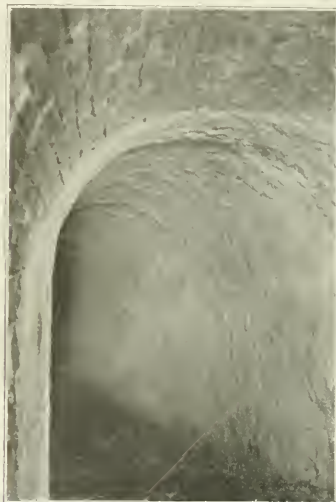
INTERIOR VIEW OF FERRY STREET SEWER, ST. LOUIS, SHOWING OLD SURFACE BEFORE AND AFTER LINING WITH CEMENT GUN MORTAR.
