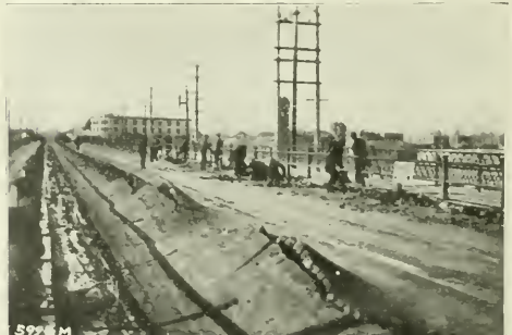
FIG. 3. A WOOD BLOCK PAVEMENT THAT BUCKLED. TROUBLE CAUSED BY EXPANSION OF THE WOOD DUE TO ABSORPTION OF WATER.
