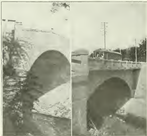
OLD STONE ARCH BUILT ABOUT 1865. ONE OF THE FEW NOT YET REPLACED BY REINFORCED CONCRETE.
