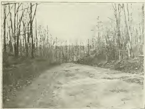
ROADWAY IN CUT NEAR ENGLEWOOD, N. J. WATER NOT KEPT OUT OR OFF. NOT WATERPROOFED. SOFTENED SPOTS WEAR INTO HOLES. RIDGES UP-HEAVED BY FROST NOT REPAIRED.
