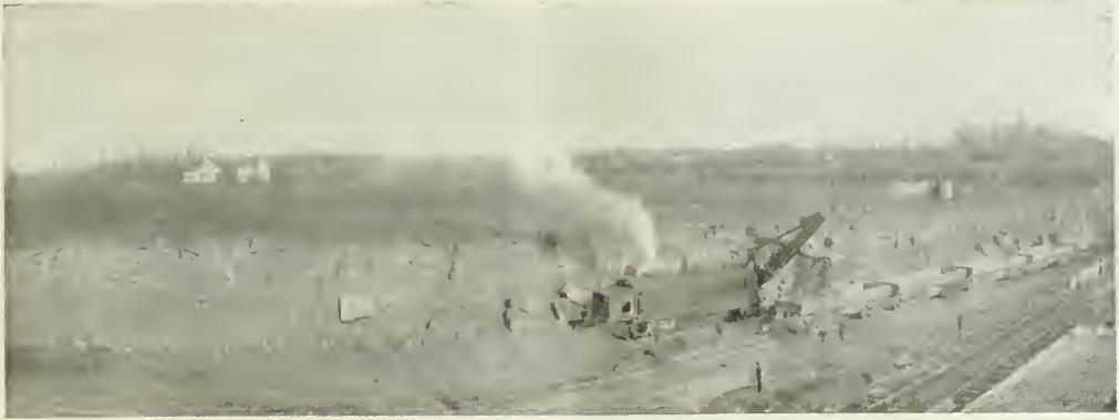
DIGGING THE SECOND CUT FOR THE BALDWIN RESERVOIR, CLEVELAND, OHIO. (THE FRED R. JONES CO., CONTRACTORS.) 100-C BUCYRUS LOADING 30-YARD WESTERN CARS. NOTE THE CHARACTER OF THE MATERIAL. THE UPPER CUT HAS BEEN COMPLETED. THE 7-FOOT BENCH MAY BE SEEN IN BOTH LOWER CORNERS. THIS BENCH CARRIES THE RUN-AROUND TRACK. CONNECTION WITH THE LOADING TRACK IN THE PIT IS MADE AT BOTH ENDS.
