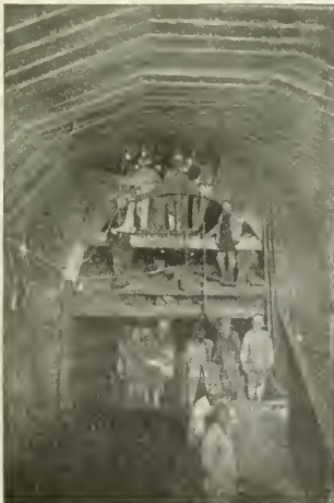
12x12 TIMBERS SET "SKIN TO SKIN," AND BEGINNING OF THE BRICK LINING IN SOFT GROUND SECTION.
