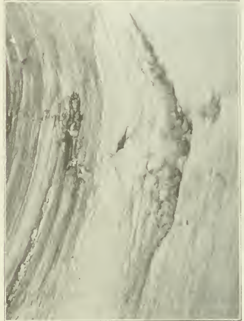
SURFACE COMPLETELY COVERED WITH DISSOLVED LIME. CRACKS IN SIDES AND DISINTEGRATION.
