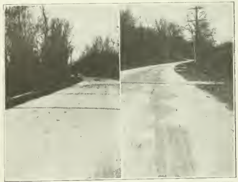
CONCRETE ROAD NEAR PLAINFIELD, N. J., WITH SOFT ASPHALT TOP. BADLY DRAINED ROAD BED. RUTTED SURFACE.
