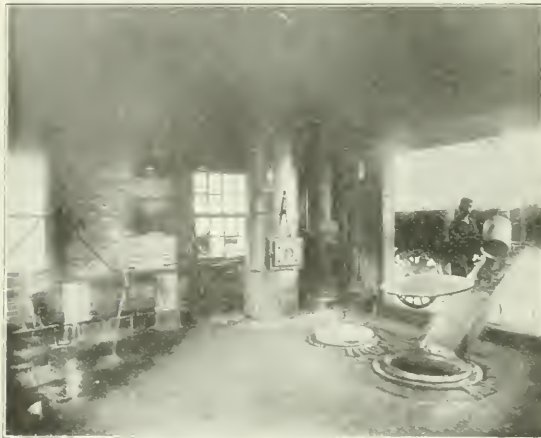
SEWICKLEY GARBAGE SYSTEM. SHOWING METHOD OF EMPTYING CANS FROM WAGON INTO CHARGING HOPPER OF INCINERATOR. TWO CHARGING HOPPERS IN FLOOR IN FOREGROUND. HOT WATER HEATER IN CORNER. FOUR OF THE FIVE CAN WASHERS AT LEFT OF PICTURE. TWO CANS ON THE WASHERS AND TWO WASHERS EXPOSED.
