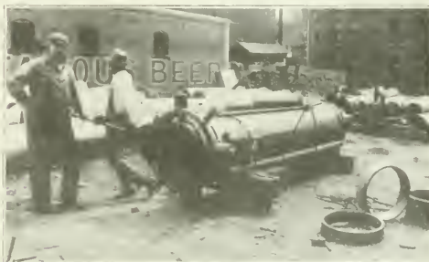
CUTTING DAMAGED ENDS OFF OF FOUR CARLOADS OF 20-INCH CAST IRON PIPE WITH A NO. 7 STRICKLER CUTTER—THREE MEN ON THE MACHINE. NOTE THE PIECES CUT OFF. PERFECT CUTS MADE ON ANY PIPE 3/4 IN. TO 30 IN.
