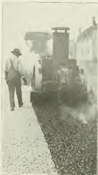
MOTOR DISTRIBUTER APPLYING BITUMEN TO SURFACE OF ROLLED BROKEN STONE LAYER IN CONSTRUCTION OF BITUMINOUS MACADAM PAVEMENT.
