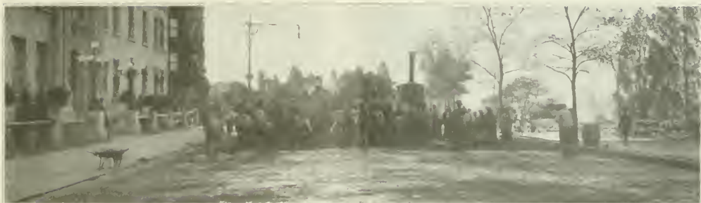
LAYING BERMUDEZ ASPHALT CONCRETE ON RIVERSIDE DRIVE, NEW YORK, ON CONCRETE FOUNDATION. TWO LAYERS OF 1½ INCHES EACH TO INSURE PERFECT COMPACTION.
