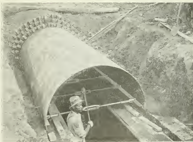
STANDARD HALF-ROUND SEWER FORMS USED ON 42-INCH TO 72-INCH BRICK SEWERS ON ATLANTA, GA., CONTRACTS BY C. W. LANE & CO. BLAW TYPE.
