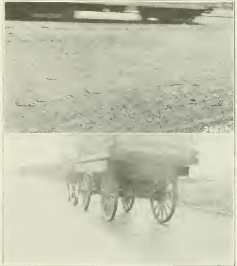
FIG. 1. BLEEDING ON A HEAVY TRAFFIC STREET. THE OIL AND FILLER COLLECTED IN LARGE MASSES WHICH ARE PICKED UP BY THE TRAFFIC.
