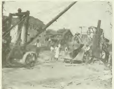
CHARGING TRACTION PAVING MIXER SKIP ON STREET WORK. GERMAN ROCK ASPHALT CO., BUFFALO, N. Y.
