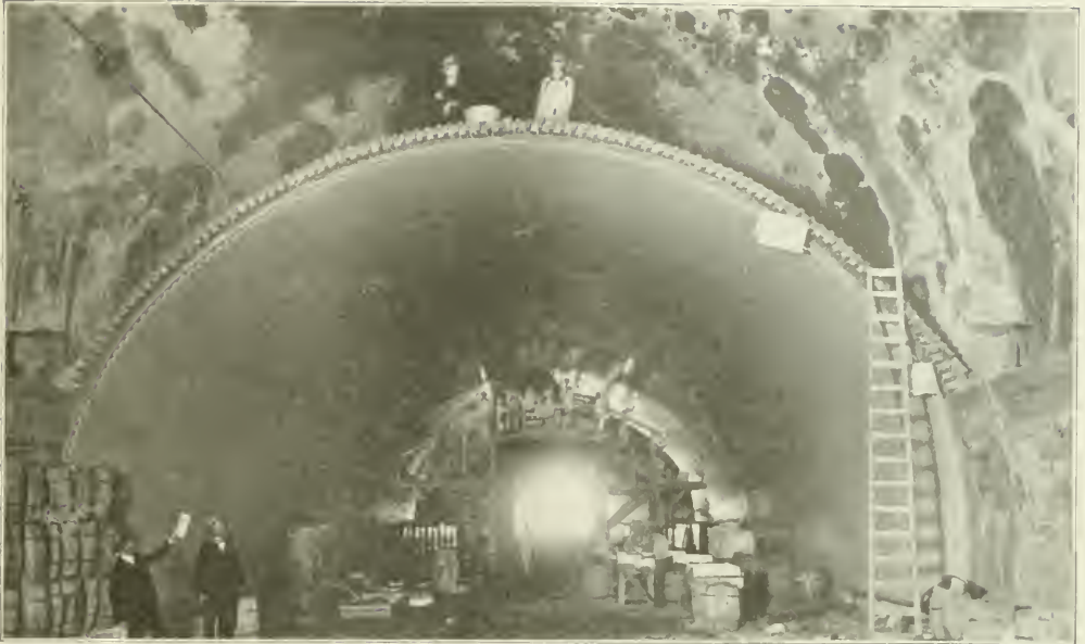
PLACING AND LINING NEW ARCH IN RECONSTRUCTING NORTH BROADWAY TUNNEL, LOS ANGELES, CALIFORNIA.
