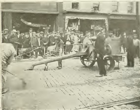
GROUT MIXER AND DISTRIBUTOR FILLING JOINTS IN A GRANITE BLOCK STREET. BROOM-MEN AT THE LEFT INSURE THAT THE JOINTS ARE FILLED FLUSH.
