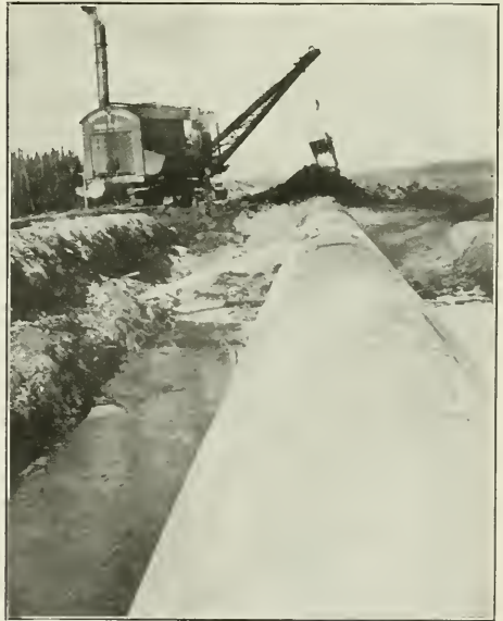
MAKING THE EMBANKMENT which covers the conduit at least four feet deep. The drag-line excavator used on some of the contracts was very successful in this sort of work.
