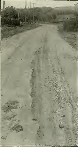
Forest Lawn Road, Florence, Neb., showing condition of road before the use of "Tarvia-X"
