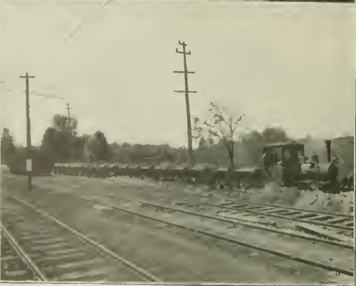
WASHING PLANT AND TRAIN, AS USED BY CONTRACTORS ON OAKLAND COUNTY, MICH., CONCRETE ROADS. CENTER VIEW SHOWS COMPLETED PAVEMENT ON WOODWARD AVE., BETWEEN ROYAL OAK AND BIRMINGHAM.
