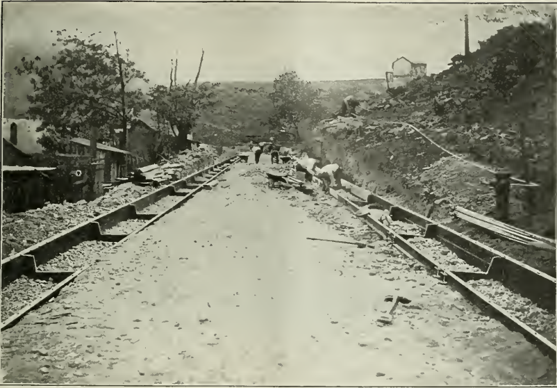
SHOWING TWO 6-INCH RAILS ON BACK OF CURB AND SINGLE 6-INCH RAIL FOR FRONT OF GUTTER. PIETRO PAVING AND CONSTRUCTION COMPANY, MORGANTOWN, W. VA., CONTRACTORS.
