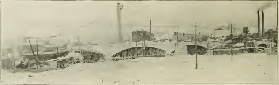
WEST WASHINGTON STREET BRIDGE UNDER CONSTRUCTION. EXCAVATION OF NEW RIVER CHANNEL IN FOREGROUND.
