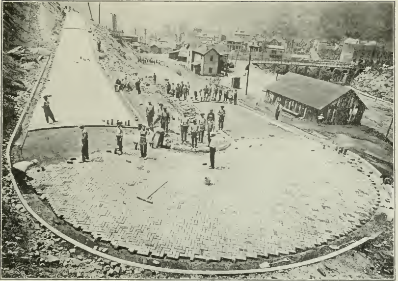
CURVED AND STRAIGHT CURB AND GUTTER CONSTRUCTION BY TILE PIETRO PAVING AND CONSTRUCTION COMPANY OF MORGANTOWN, W. VA.
