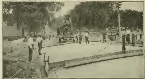
CEMENT PAVING AT LAKE MILLS, WIS., MADE PERFECT THROUGH USE OF ROUGHEN GAGE. ALSO USED AS A BRIDGE.
