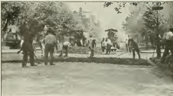
LAYING TOPPING BEHIND LUTZ SURFACE HEATERS, 1,200 SQUARE YARDS LAID IN AN EIGHT-HOUR DAY.
