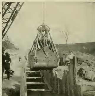
FIG. 1. SEWER TRENCHES MAY BE EXCAVATED WITH HAYWARD BUCKETS AND THE MATERIAL LOADED DIRECTLY INTO WAGONS, WITHOUT THE AID OF A HOPPER. THE ILLUSTRATION SHOWS A TRAVELING DERRICK OPERATING IN THIS WAY.
