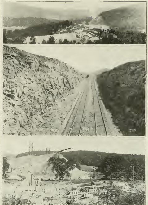
VIEWS showing the extent of cuts and fills where they were chosen instead of viaduct construction.
