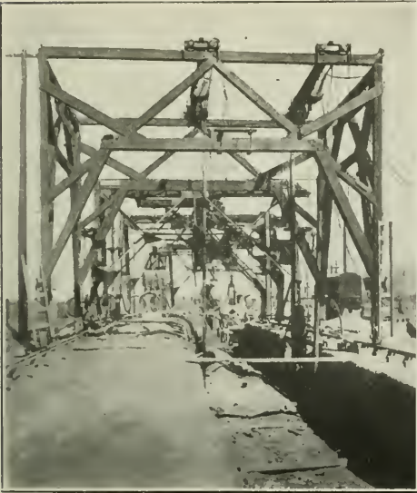
TRAVELER WITH ELECTRIC MACHINERY spanning sewer trench. In foreground sheet piling is handled and driven by two electric hoists on two small travelers. In the rear are the digging and pipe-laying cranes with hoists for handling the orange-peel or clamshell buckets and the sections of pipe to be laid. The portable sub-station is seen on the right.
