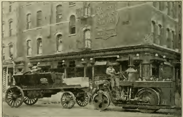
VIEW SHOWING FIVE-TON ROAD ROLLER HAULING 120-CUBIC-FOOT TRAILER FROM PATCH TO PATCH ON ASPHALT REPAIR WORK.
