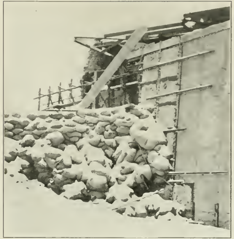
WHEN THE USUAL JANUARY FLOOD CAME THIS WINTER THIS SECTION OF THE WALL WAS NOT COMPLETED. THE GAP WAS FILLED WITH SAND BAGS AND GRAVEL AND THE WATER WAS KEPT OUT, EXCEPT A LITTLE SEEPAGE, ALTHOUGH IT CAME UP ALMOST TO THE TOP OF THE PILE OF BAGS SHOWN. THIS VIEW WAS TAKEN ON THE RIVER SIDE OF THE WALL.
