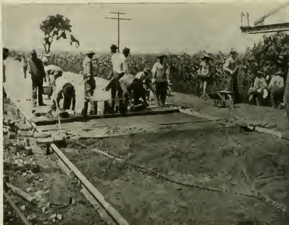
LAYING THE BRICK on the Middle Springfield road, Paris, Ill., monolithic brick pavement construction.
