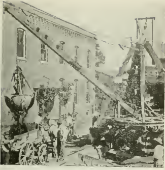
FIG. 2. HAYWARD BUCKETS ON SEWER WORK. WITH THE TRENCH MEASURING 6 FEET WIDE AND THE SPACE BETWEEN AVERAGING 10 FEET, THIS 1\frac{1}{2} -CUBIC-YARD BUCKET DUG ALL GRADES OF SAND, LOAM AND GRAVEL.
