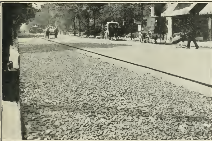
Peachtree street, looking south from Tenth street. Stone base being rolled to grade before coating with asphaltic cement.
