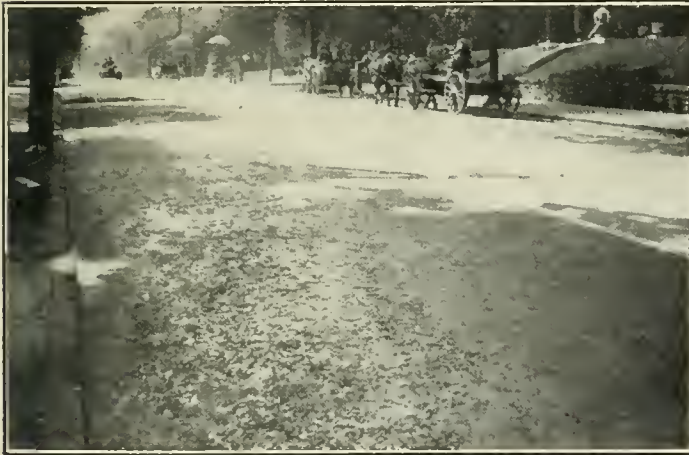
Peachtree street, looking toward Peachtree Place. Top course of bitulithic surface being placed; taken before rolling.
