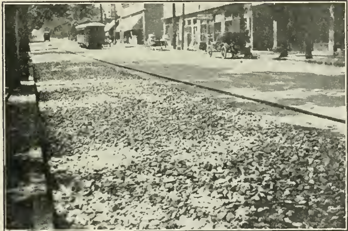
Peachtree street, looking south toward Peachtree Place. Foundation of eight inches of stone, rolled to grade and covered with asphaltic cement.
