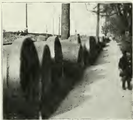
THIRTY-THREE-INCH vitrified sewer pipe ready for installation in Chicago suburb. Shown through courtesy of Blackmer & Post Pipe Company, St. Louis, Mo.
