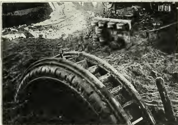
INTERIOR view of power house, Black River Falls, Wis., May 21, showing electrical equipment buried beneath tons of sand and other debris.
