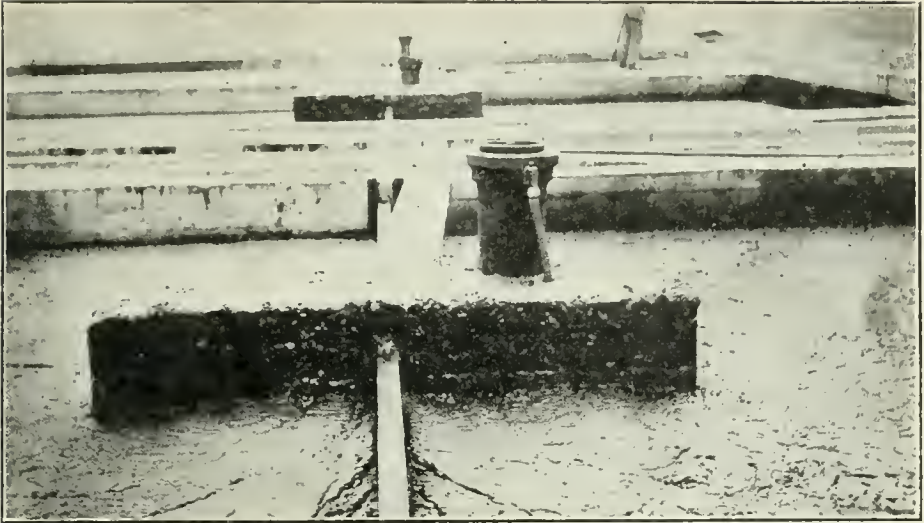
III. THE SLUDGE in the digesting tank below has foamed up and over out of the openings from that tank to the air, and is spreading over the water in the upper tanks and over the ground. This action is stopped by drawing off the sludge from below.
