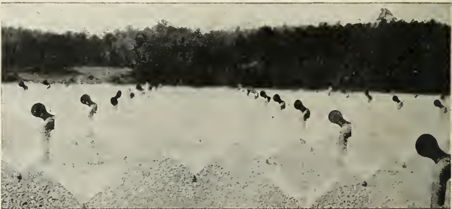
390 TAYLOR NOZZLES at Atlanta, Ga., operated by two 24-in. Miller Sewage Siphons.
