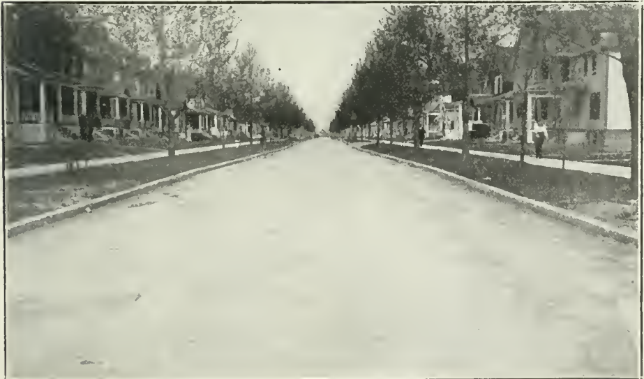
CONCRETE PAVEMENT, Detroit, Mich. General condition excellent. Note perfect steel-protected joints. Spot on left is a cut, temporarily filled with earth and planks on top. Note level street, with straight grade at center and breaks in curb grades to give drainage for gutters.
