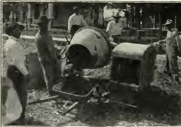
"BIG-AN-LITTLE" concrete mixer in use at Dallas, Tex., for construction of concrete curbs and gutters.
