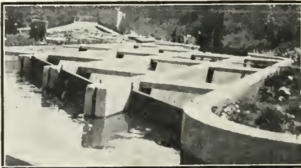
G RIT CHAMBER, Peachtree Creek Sewage Disposal Plant, Atlanta, Ga.
