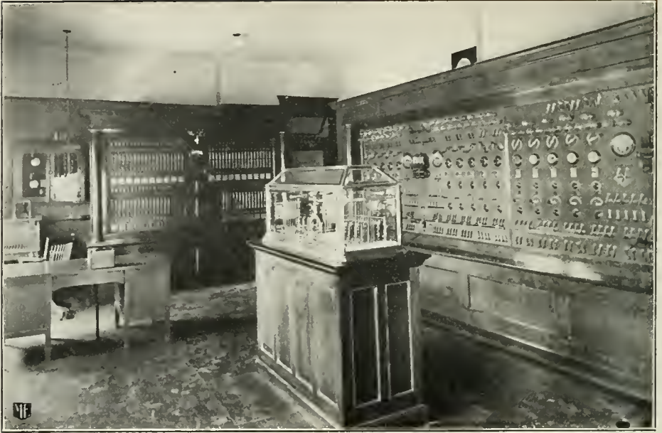
S WITCHBOARD room at central fire station, Fort Worth, Texas—the most important link in a system which was carefully planned and has been notably successful. Shown by courtesy of the Fort Worth Star-Telegram.
