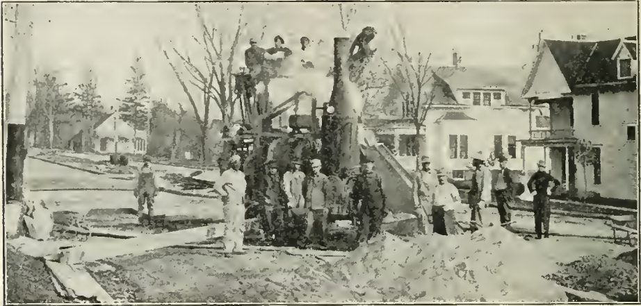
STREET paving in Clarinda, Ia., work being done by the Concrete Construction Co., Cedar Rapids, Koehring street paving mixer in foreground.
