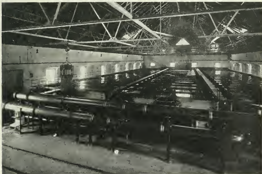
I NTERIOR of the filter house showing piping in foreground; filter beds in the rear and cleaning apparatus between.
