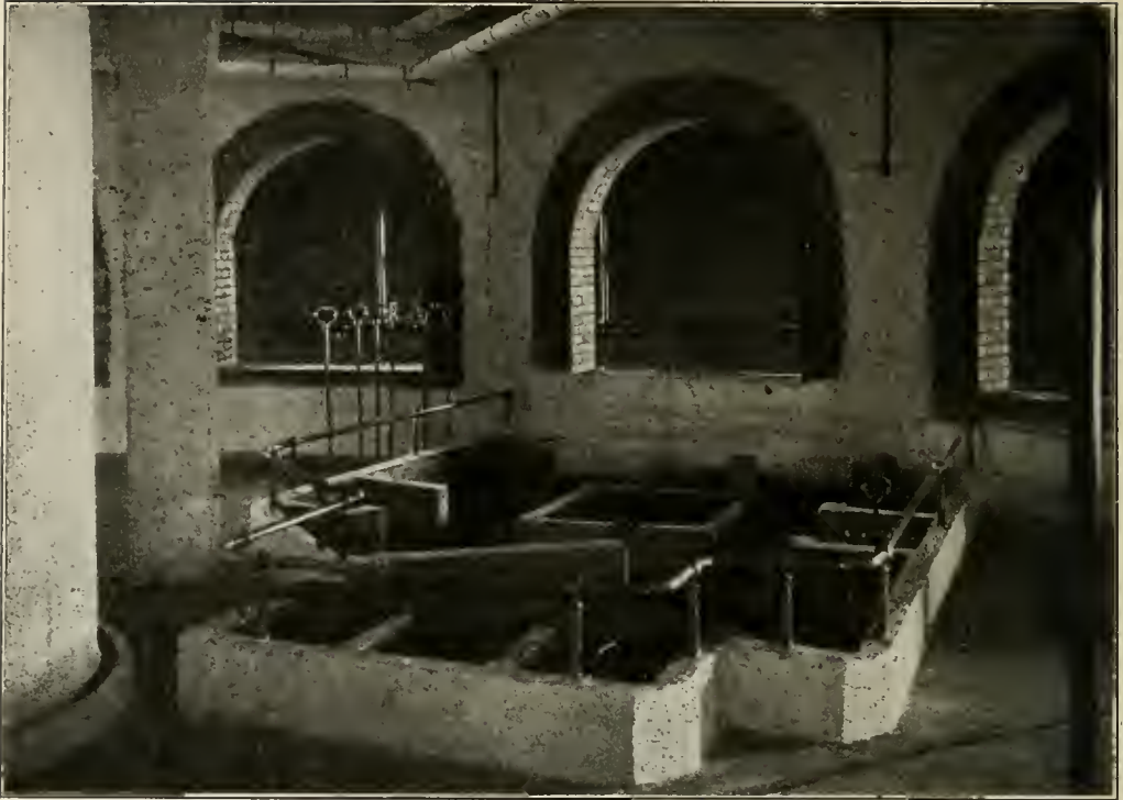
FILTER ROOM, McKeesport water purification plant.
