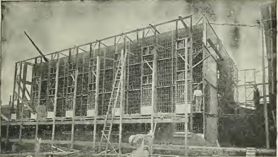
View of Cage containing 120 steel cells at the Hartford County Jail, Hartford, Conn. Erected by us before carrying up outside masonry walls.
