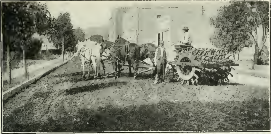
CONSTRUCTING an asphalt macadam street at Whittier, Cal. A petrolithic tamping roller is in the foreground.
