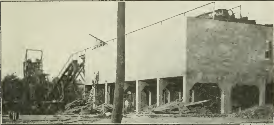
GRAVEL WASHING PLANT and its concrete storage bins, Norfolk, Va.
