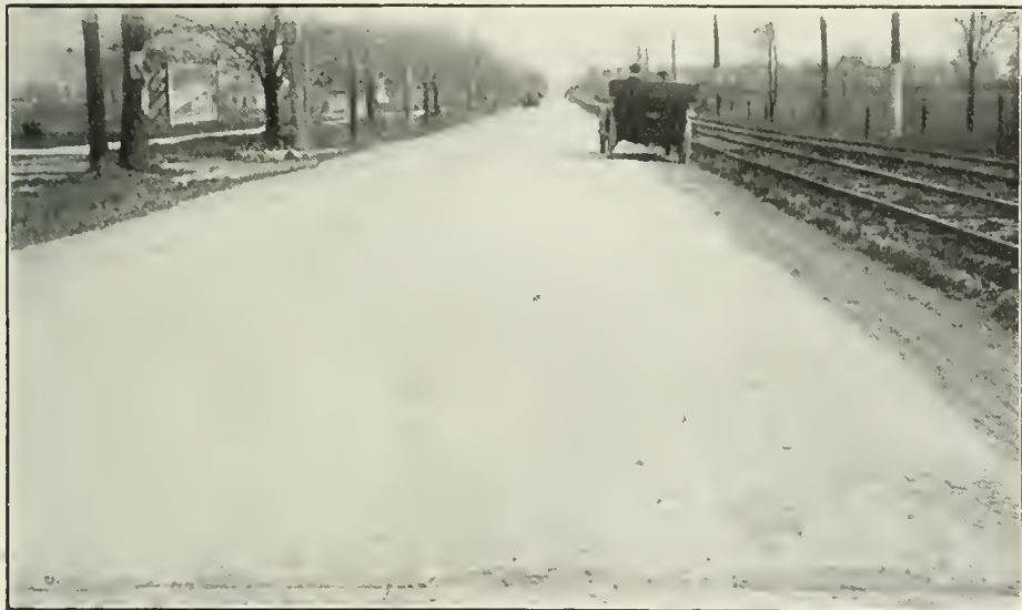
CONCRETE HIGHWAY IN WAYNE COUNTY, Michigan, about five years old, not reinforced. General condition excellent. Note longitudinal crack and one break in right-hand corner. Joint in foreground has bituminous filler.
