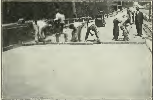
L AYING brick on Chevy Chase sample road. The two-inch sand cushion is shown in front and the roller is following closely behind the brick-laying gang.
