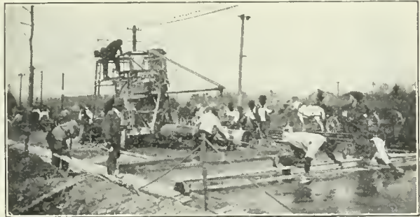
L AYING concrete direct from mixer and floating surface of Chevy Chase sample concrete road. The large portable mixer discharges the concrete exactly where it is wanted.
