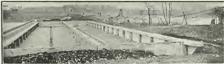
SPRINGFIELD, MO., Sewage disposal plant; filter bed ready for filling with broken stone.
