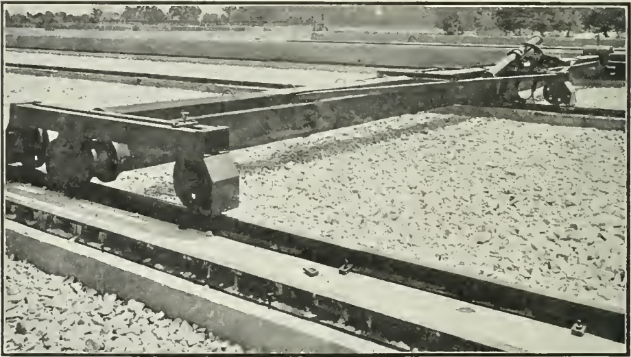
TRAVELING DISTRIBUTER, which sprinkles sewage over the bed thru perforated pipes fed from sewage trough at one end. Hauled by rope; motion reversed by "gun" at center of distributor.
