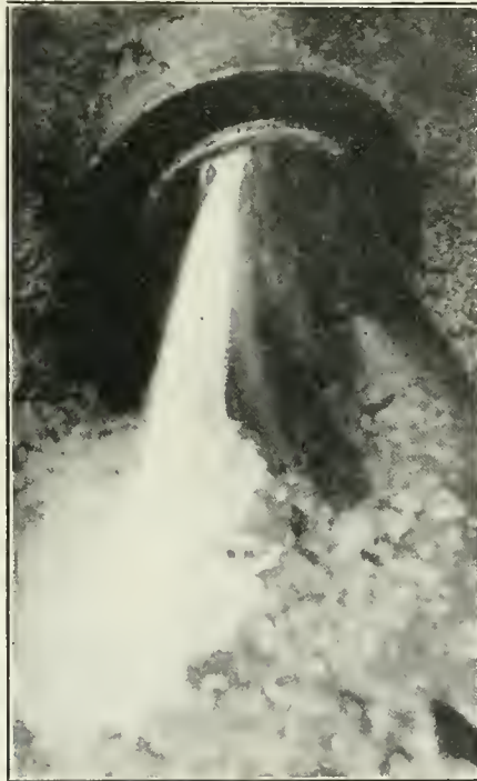
P ARTIALLY blown joint leaking 29,000 gallons a day. Leak located by Pulsograph.
