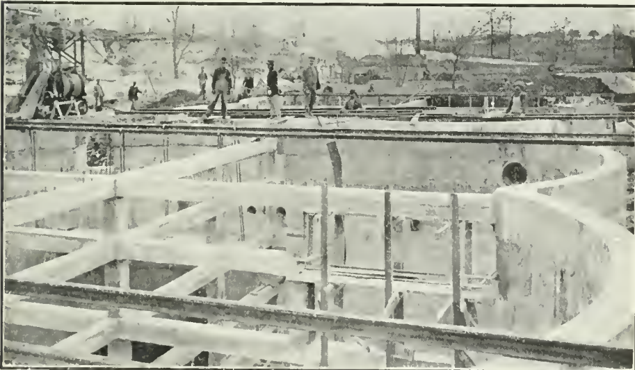
SETTLING TANKS under construction, showing the reinforced concrete streets, acting also as tie rods to take strains from the lobe-shaped walls.
