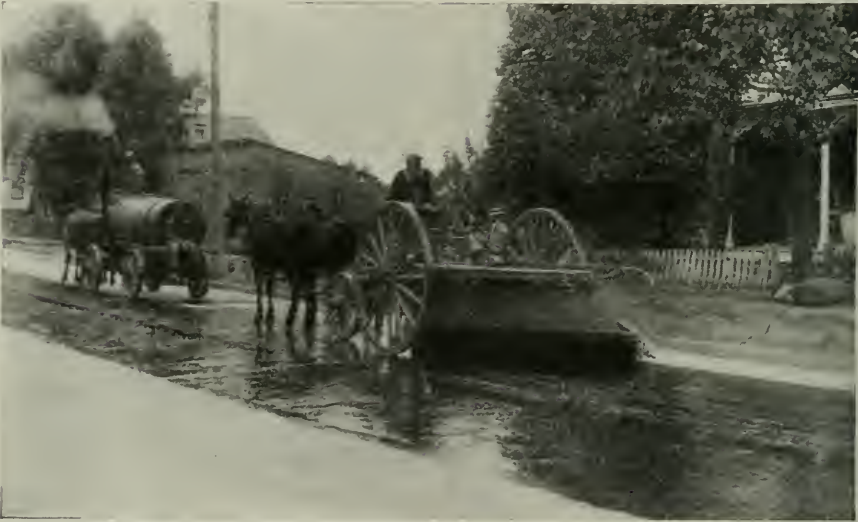
ONE OF THE METHODS OF APPLYING AND SPREADING DOLARWAY BITUMEN ON CONCRETE BASE.
