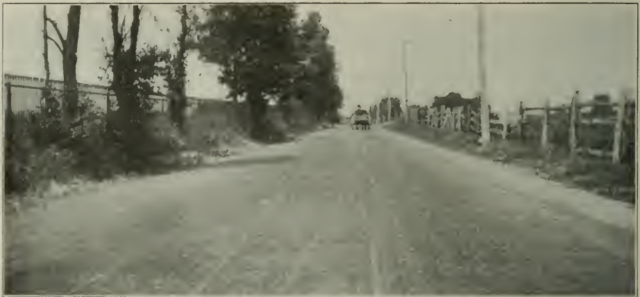
4. PARK HEIGHTS EXPERIMENTAL ROAD, BALTIMORE, MD. Section 17. Standard Asphalt & Rubber Co., Sarco
