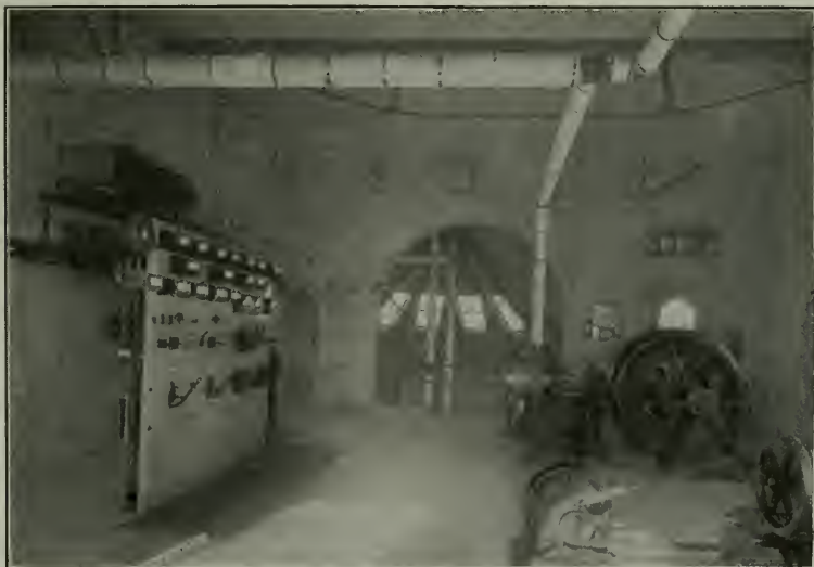
ELECTRIC LIGHT AND WATER PLANT, ST. MARYS, KANSAS. Electric Generators and Switchboard.
