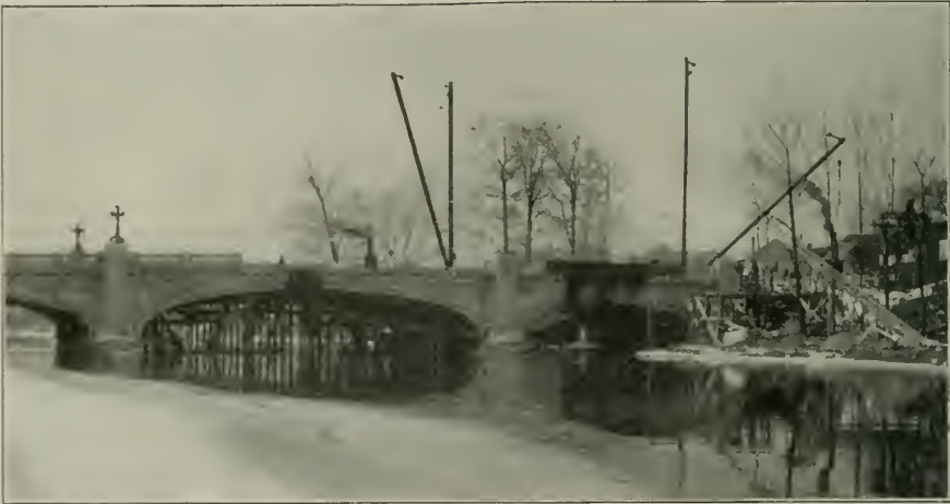
CAPITOL AVENUE BRIDGE, INDIANAPOLIS, IND North End, Showing Plant for Handling Concrete and Concrete Materials.
