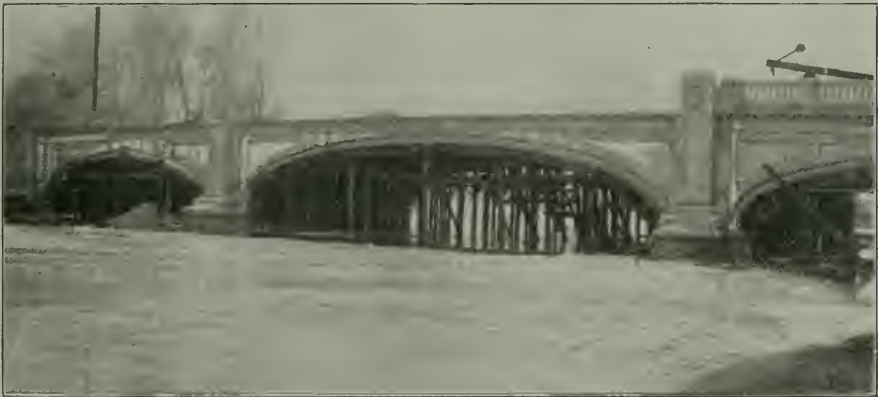
CAPITOL AVENUE BRIDGE, INDIANAPOLIS, IND. South End, Showing Centering and Completed Arches Without Parapet.
