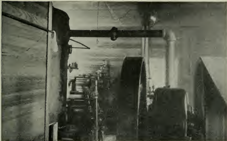
SHIRLEY, IND., PUMPING STATION AIR COMPRESSOR, TANK AND AUTOMATIC SWITCH.
