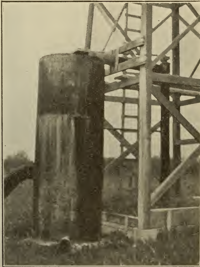
THE LOS ANGELES WATER WORKS. One of the Wells at the Slauson Avenue Station.
