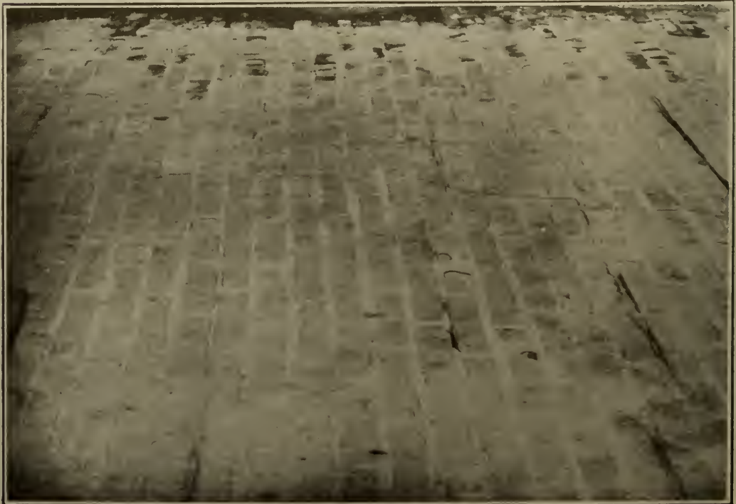
6. HARBOR STREET, CONNEAUT, O. Cement filled brick street laid in 1900 on natural soil, immediately south of L. S. & M. S. Ry.
