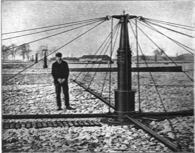
Fig. 54.—Centre Pillar of Circular Distributor, Showing Method of Supporting the Radiating Arms with Guy Ropes.
