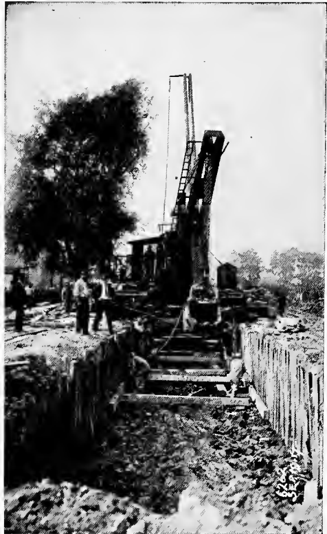
FIG. 93.—Steam Shovel at Work on Sewer Trench for North Shore Intercepting Sewer, Evanston, Illinois.
