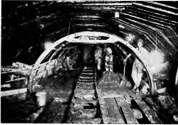
FIG. 132.—Ogier's Run Intercepting Storm-Water Drain, Baltimore, Maryland.
