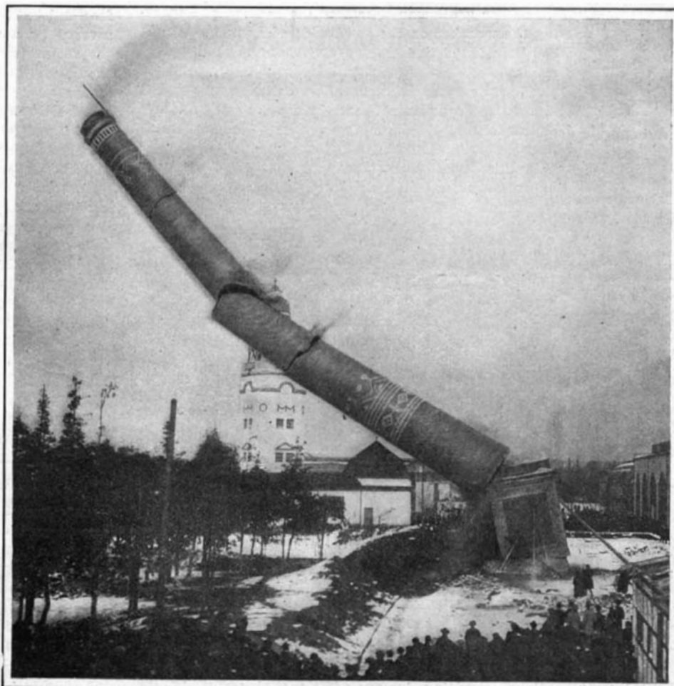
Fig. 3.—As It Fell the Stack Slid From Its Pedestal and Broke Into Several Parts.
