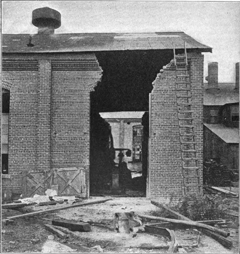
FIG. 2. THE WRECKED ENGINE ROOM.
