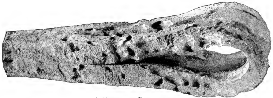
A CORRODED BRACE.
