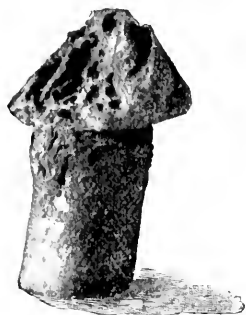
A CORRODED RIVET.
