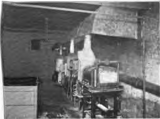
Fig. 3. View of Hardening Plant shown in Fig. 2, taken from Street End
