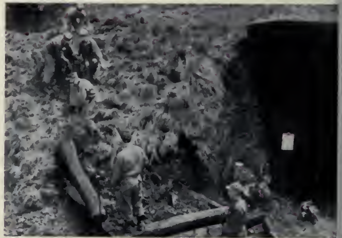
Here, the reservists begin building one of the bridges to carry pedestrian traffic to Lynch Field without having to use heavily traveled Route 119. Rights-of-way were secured from a railroad, an oil company, and a private individual.
