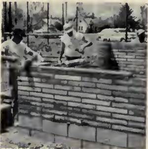
Members of local Bricklayers Union spent many free hours constructing cement-block rest room. Note first level of backstop poles.
