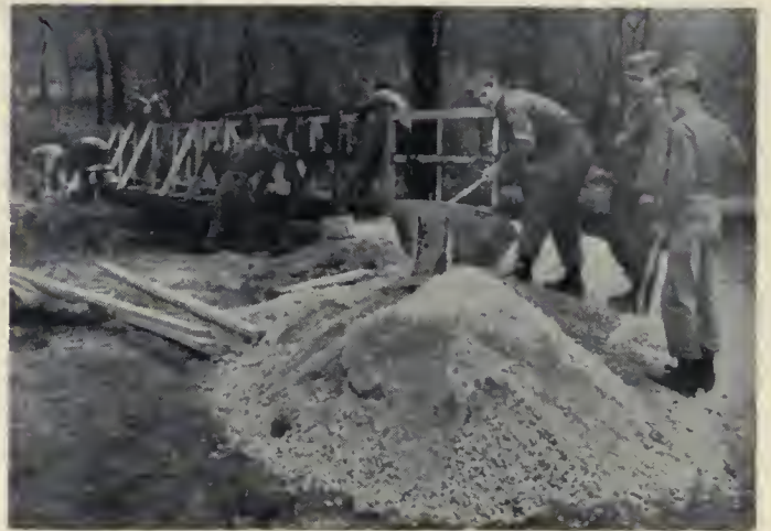
One of the bridges nears completion as reservists tighten guard rails and finish off approaches with gravel. At the far end of the bridge some of the men are cleaning up; on the near side others load gravel for approach to bridge.
