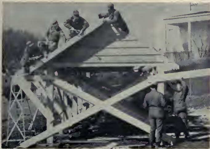
A shelter goes up! Here, the reservists assemble one of the shelters. One group tackles putting on the roof while another group works on the lower part of the building. The result is fine array of new shelters for the community.
