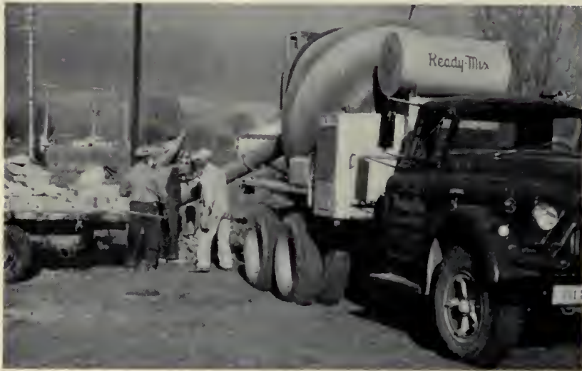
Men pour concrete for footings, floor, and backstop poles. All backstop poles were the donation of local companies.
