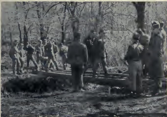
Reservists begin to lay the foundations for another bridge to the park. All material and equipment were furnished by recreation board. Army supplied manpower and professional staff. New cooperative projects are in offing.
