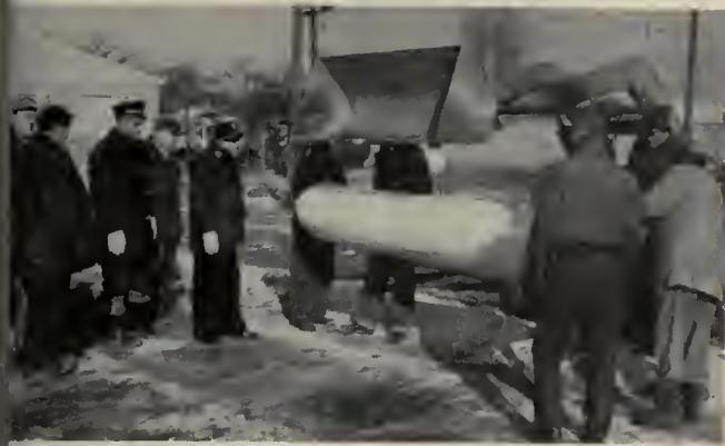
Above: The .006-mil plastic, carried on the bucket arm of a back hoe, is delivered by the public works crew. A two-inch pipe had been inserted into the core of the rolled plastic and attached by chain to a second pipe to allow the plastic to be peeled off in the spreading operation. Hole in foreground is for suction intake to be used to pump water from the rink. Water-retaining berm is made from agricultural limestone.
