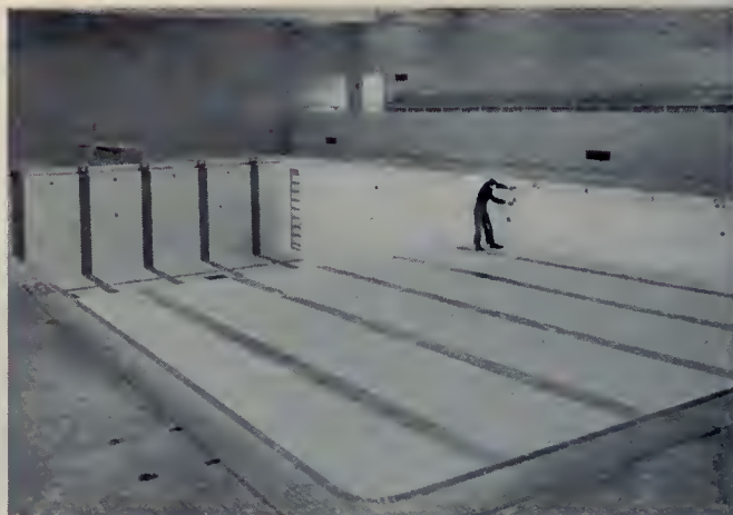
Handsome, all-ceramic tile pool in junior high school, Great Neck, New York, combines utility with attractiveness. A worker spots where safety rope will cross pool, separating diving area from shallow water. The 75-by-36-foot pool has cleat-tread tile at both ends for nonslip swim turns.
