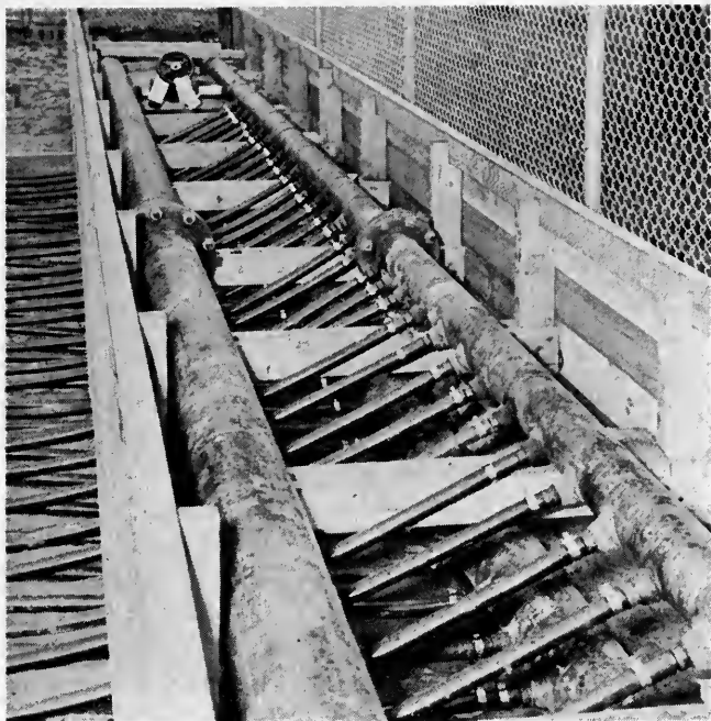
Iron header pipes, which are enclosed in a permanent installation, conduct brine to plastic tubes in Detroit's take-up rinks. These tubes can be rolled up and stored.
