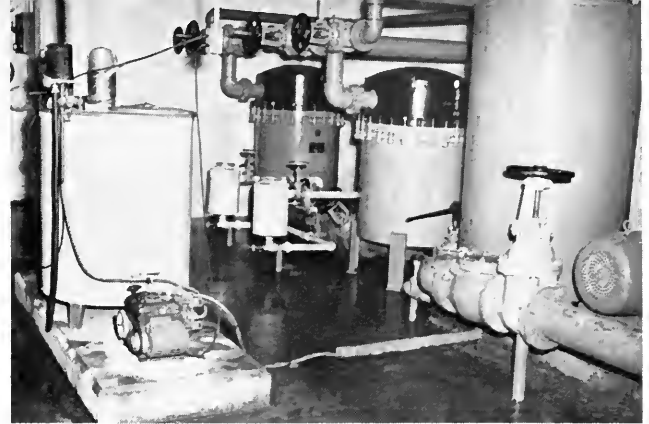
No Help Wanted! This bit of machinery does everything necessary to the 97,000 gallons of water the pools hold. Chlorine count, water level, and the water's purity are maintained around the clock without a single finger ever being lifted. Tank on left is chlorinator. Large tank in the foreground mixes the water, maintains water level.
