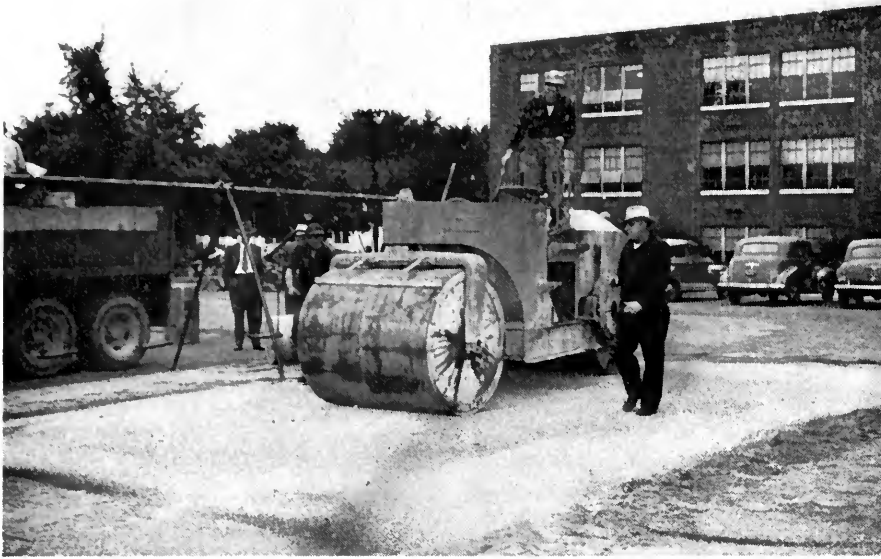
Under pressure of the roller, rubber particles and fluid asphalt are forced together. Mechanical spreading equipment helps effect uniform distribution.
