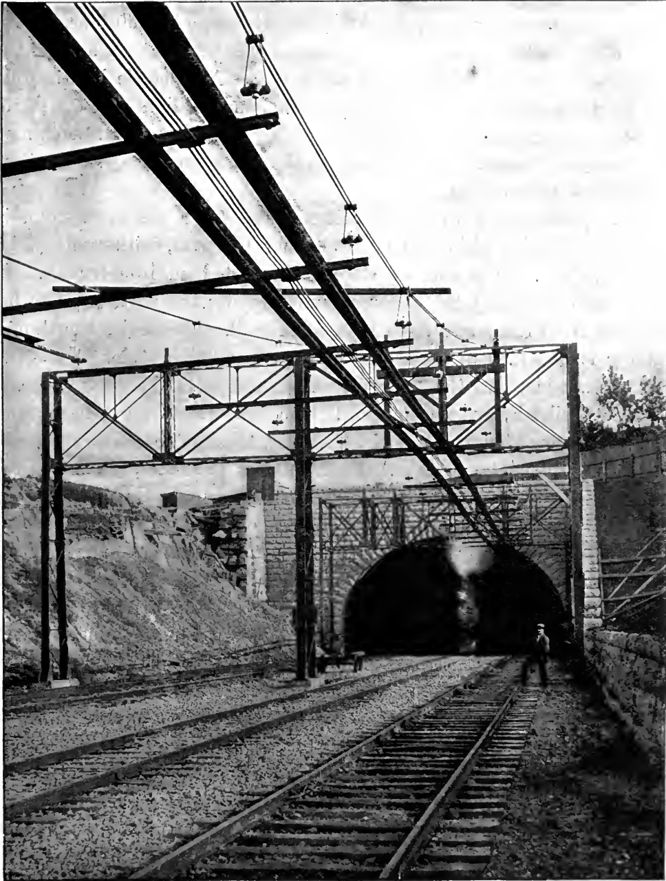
FIG. 330. ELECTRIC CONDUCTORS AT PORTAL OF THE BALTIMORE TUNNEL.
