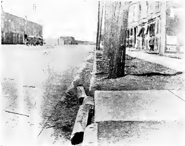
RESULT OF BUILDING CONCRETE CURB DIRECTLY ABUT- TING AGAINST WALK.
