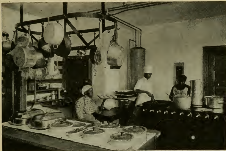
Commercial electric range installation in a large apartment house kitchen in the South. Colored people, too, delight in cooking electrically. The steam table in the foreground is also electrically heated.
