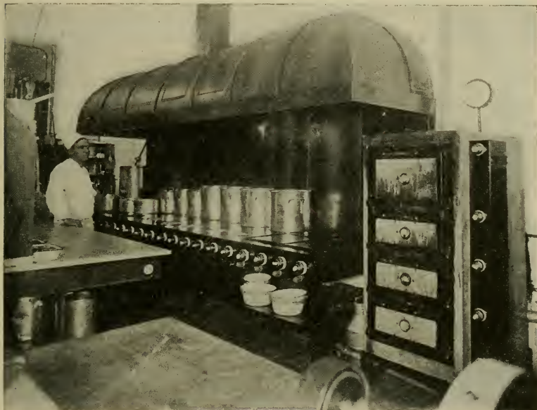
Complete electric kitchen installed in a large cafeteria in the West. Note the small space occupied by the electric oven which does all the baking for this large restaurant.
