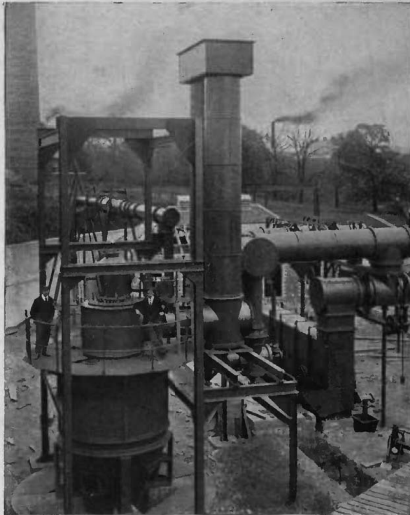
VIEW OF THE MOND GAS PLANT AT THE WORKS OF THE UNITED TURKEY RED COMPANY, LTD., ALEXANDRIA, NEAR GLASGOW, SCOTLAND, (SHOWING THE WATER-SEAL TO THE PRODUCER).
