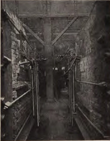
Fig. 79. Water-Cooled Burners Applied to Open Hearth Furnace.
