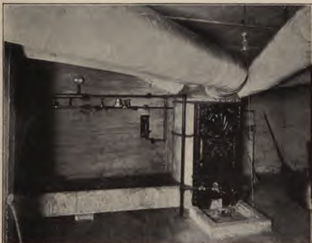
Fig. 96. Heating Furnace in Officers' Quarters.
