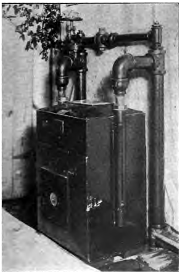
Fig. 271. Unusual Installation of Dry Meter
