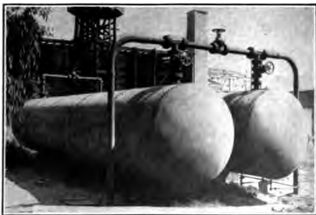
Fig. 119. Pressure Storage in California
