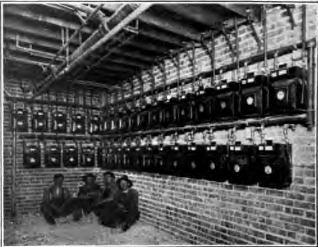
Fig. 274. Well-Arranged Installation of Tin Meters
