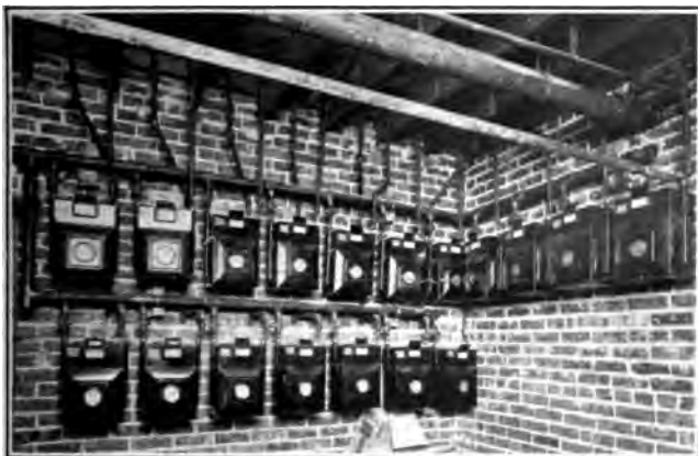
Fig. 273. Apartment House Bank of Dry Meters
