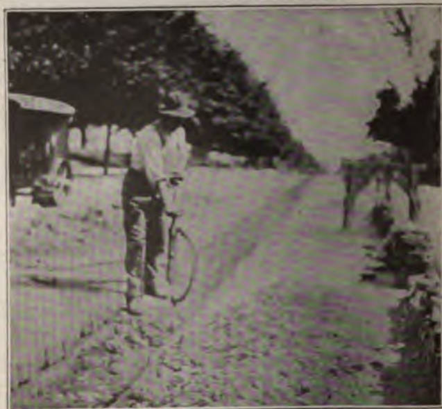
Fig. 159. Quicker and Easier Than Picks, Sledges and Bars minute, depending on the character and hardness of the soil and the size of the trench.
