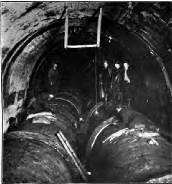
Fig. 4. Modern Installation of Gas Mains in Tunnel
