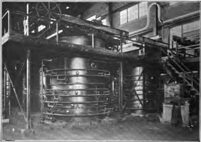
FIG. 355.—Battery of surface combustion heat treating furnaces for quenching and drawing cannon tubes, Watertown Arsenal. Boston city gas used as fuel.
