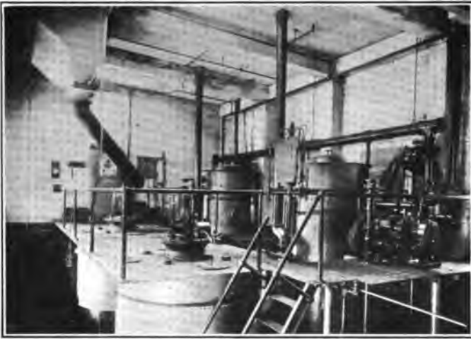
FIG. 287.—Two 100-hp. units, anthracite heat, for hardening, tempering, etc., Simonds Canada Saw Company, Montreal, P. Q.
