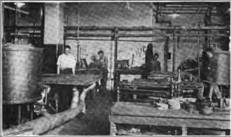
FIG. 360. —Battery of surface combustion lead-melting furnaces for continuous melting in an electrotype shop. City gas used as fuel.
