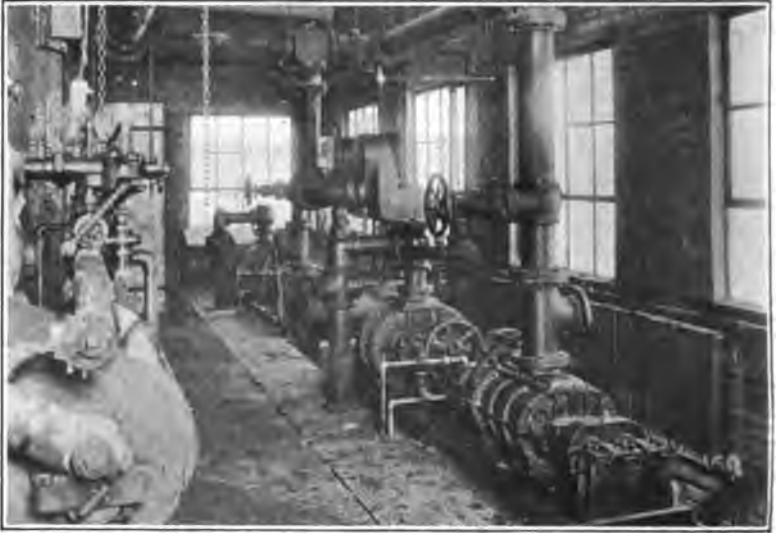
FIG. 323.—Compressor, exhauster, and tar extractor equipment installed at the Aluminum Castings Company, Cleveland, Ohio.
