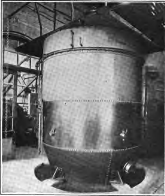
FIG. 294.—Three hundred-hp. anthracite, 250-hp. for engine, d. c. to generator, balance of gas used for hardening, annealing, etc. ( Keystone Watch Case Company, Jersey City, N. J. )
