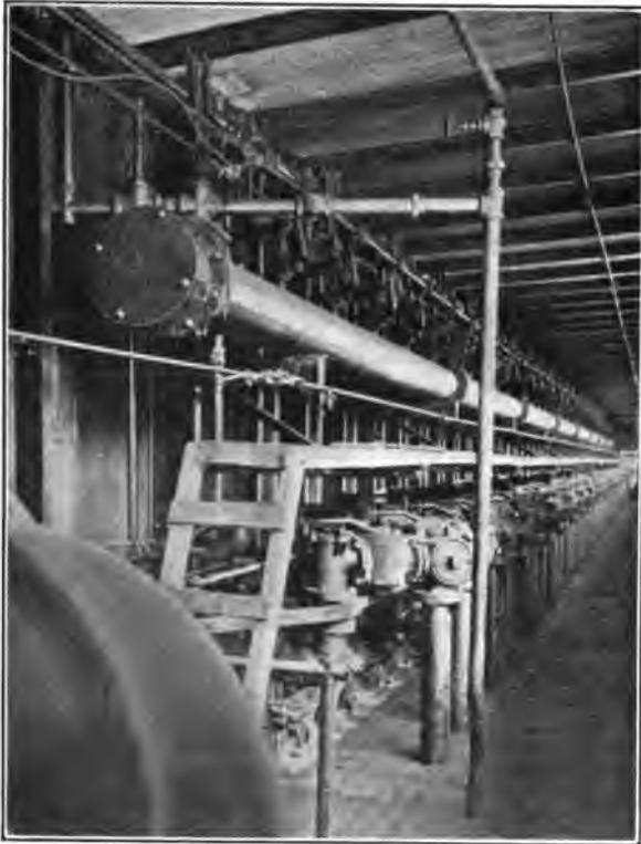
FIG. 45.—Arrangement for firing Koppers combination ovens with either producer gas or coke-oven gas.
