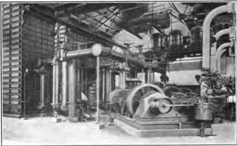
FIG. 47.—Gas washers, tar extractors and exhausters for indirect process installed by The Koppers Company for the Laclede Gas Light Company, St. Louis, Mo.
