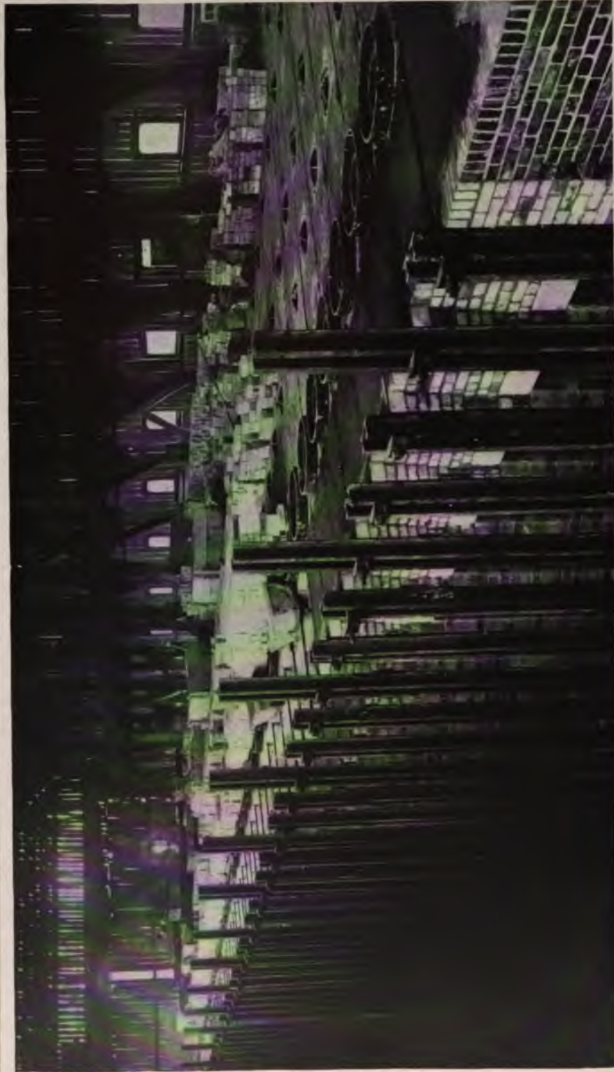
FIGURE 55. VIEW DURING CONSTRUCTION OF 50 ADDITIONAL UNITED-OTTO OVENS AT THE CAMDEN PLANT, JANUARY 13, 1906.
