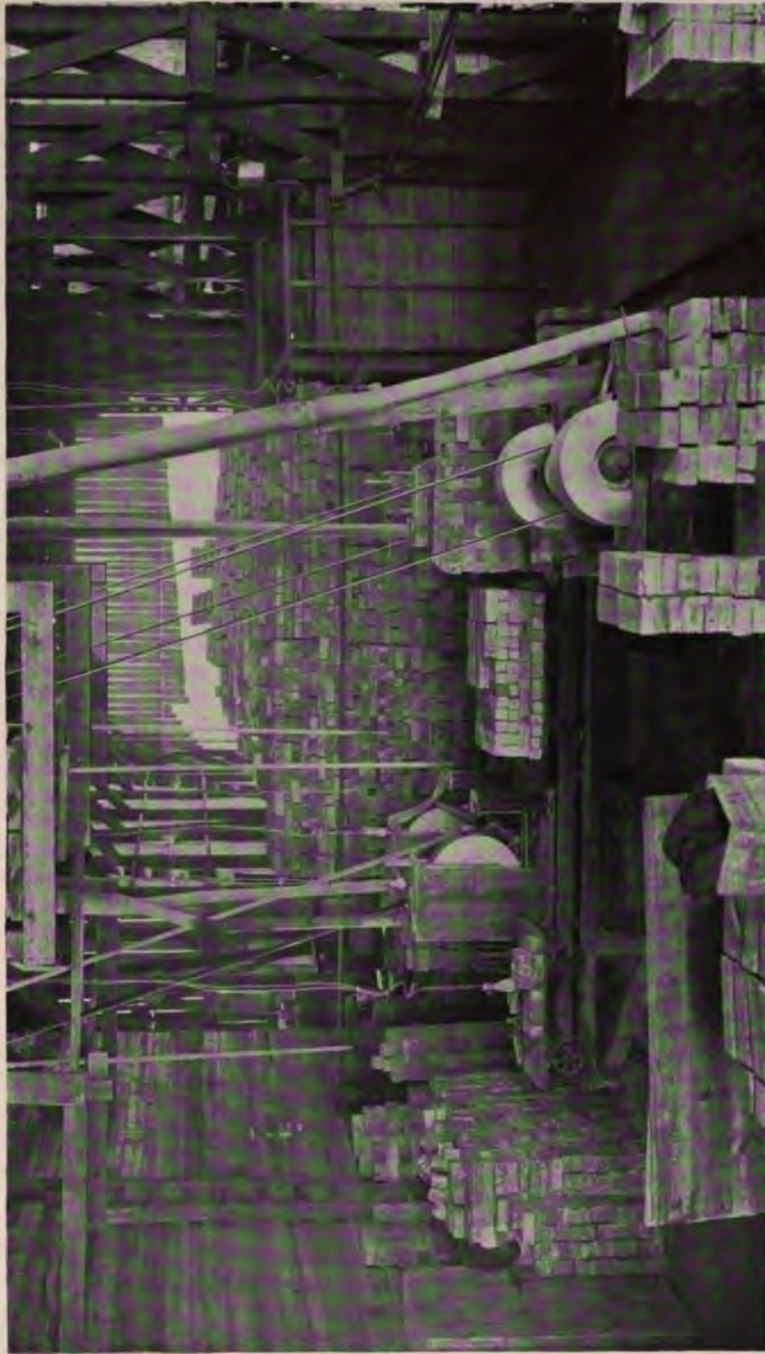
FIGURE 54. VIEW DURING CONSTRUCTION OF 50 ADDITIONAL UNITED-OTTO OVENS AT THE CAMDEN PLANT, NOVEMBER 1, 1905.
