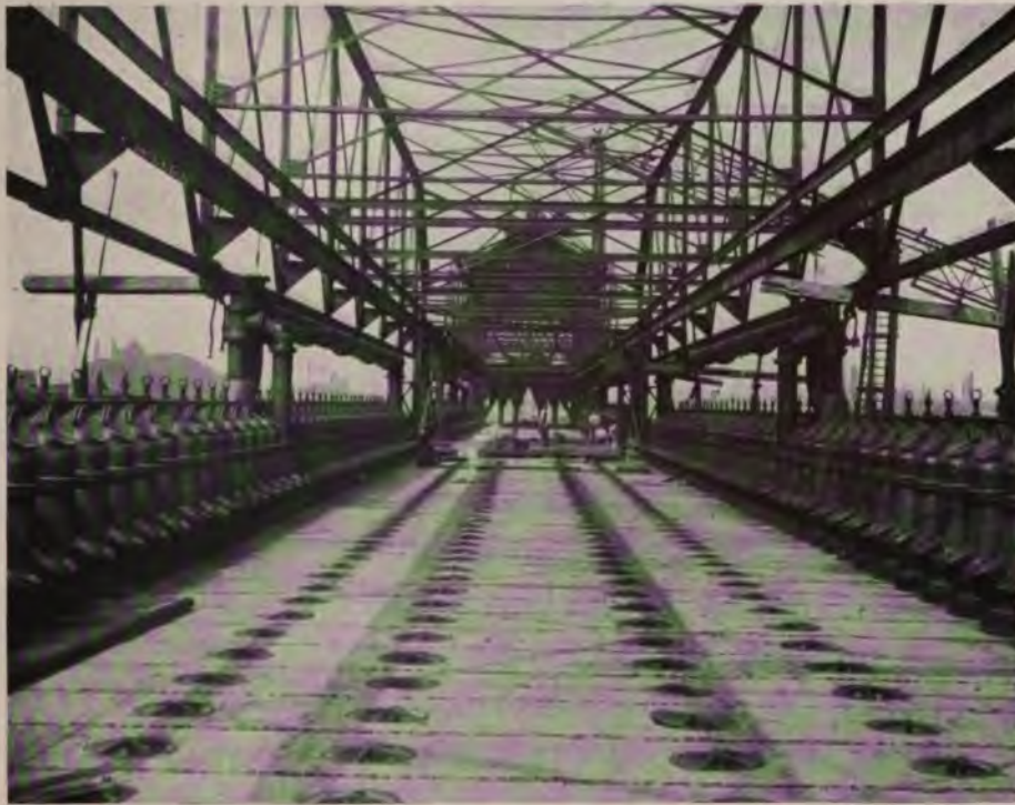
FIGURE 15. ELECTRICALLY OPERATED CHARGING LARRY AND SUPPORTING BRIDGE AT THE CAMDEN PLANT.
