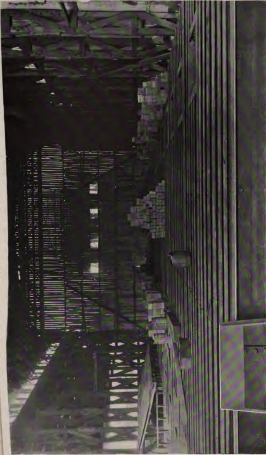
FIGURE 53. VIEW DURING CONSTRUCTION OF 50 ADDITIONAL UNITED-OTTO OVENS AT THE CAMDEN PLANT, OCTOBER 7, 1905.
