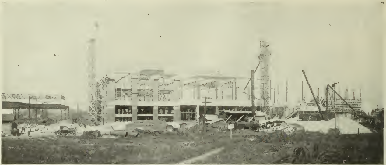
New Foundry of General Fire Extinguisher Co., Warren, O. Designed by The H. M. Lane Company
