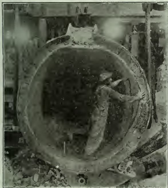
Relining a 40-ton ladle in steel foundry using Hytempite for laying up and surfacing.
