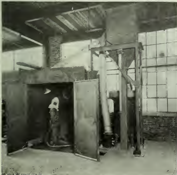
Sand Blast Room Installed in the New Plant of the Cleveland Cooperative Stove Co.
