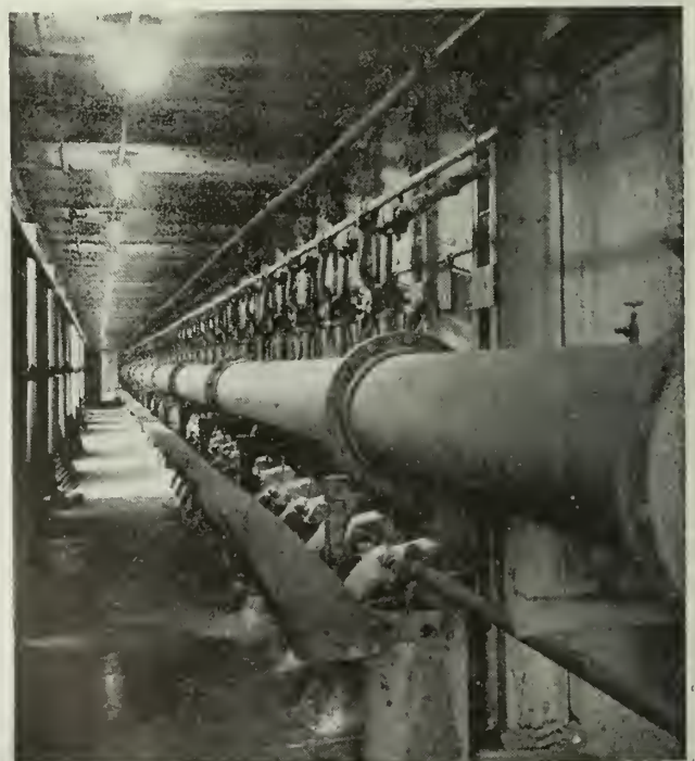
ONE OF THE GAS MAINS ON THE COKE OVENS SHOWING THE RISERS AND VALVE CONTROL.
