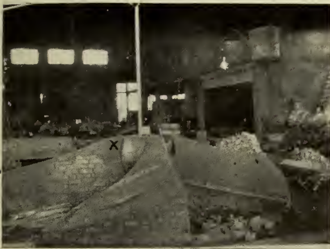
FIG. 5.—DRIVING SURFACES SWEEPED UP AND THICKNESS PIECES IN POSITION. NOTE DRAW BACK MARKED "X."
