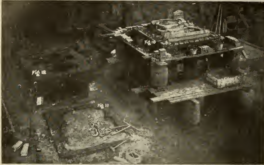
FIG. 10. INTERMEDIATE CYLINDER MOLD WITH BRICK WORK NEARING COMPLETION. FIG. 11. LIFTING PLATE FOR SEPARATING THE MOLD AND ALSO FOR SUPPORTING IT AGAINST THE STRAIN OF THE METAL. FIG. 12. COVER FOR INTERMEDIATE CYLINDER.
