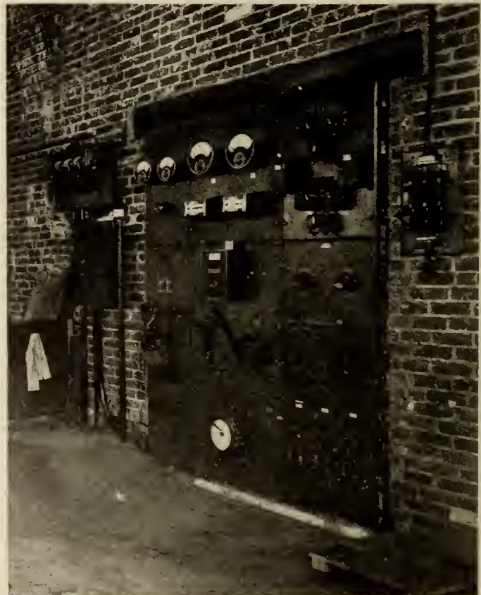
SWITCHBOARD AND AUTOMATIC ELECTRODE CONTROL.
