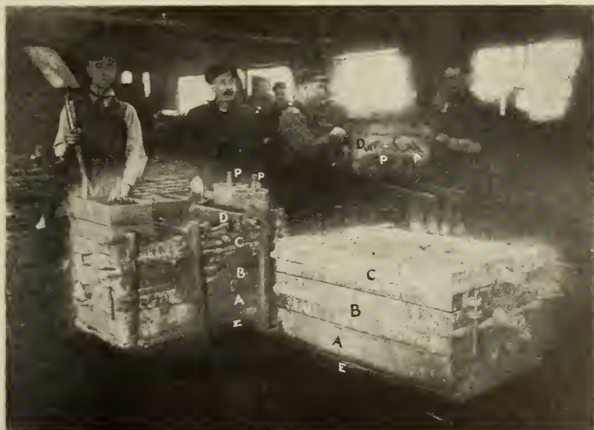
FIG. 4—TO LEFT, BUILDING, POURING BASIN AND RISERS. TO RIGHT, WORKMEN CLOSING ON SMALL COPE.
