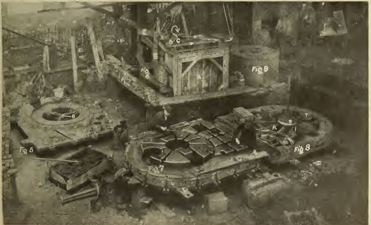
FIG. 5—FOUNDATION PLATE ON WHICH MOLD IS BUILT. FIG. 6 IS MOLD FOR FIG. 3 IN PARTLY BUILT UP. FIG. 7 IS COVER OR COPE FOR MOLD FIG. 3. FIG. 8 IS FALSE COPE OR PATTERN ON WHICH TO BUILD FIG. 7. FIG. 9 IS MAIN BARREL-CORE FOR L.P. CYLINDER.
