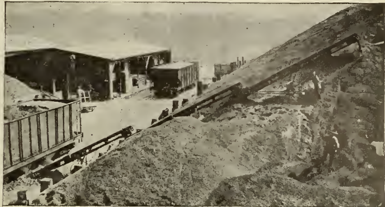
FIG. 5—USING THREE SCOOP CONVEYORS TO UNLOAD FROM HOPPER BOTTOM CARS TO LARGE STORAGE PILE.
