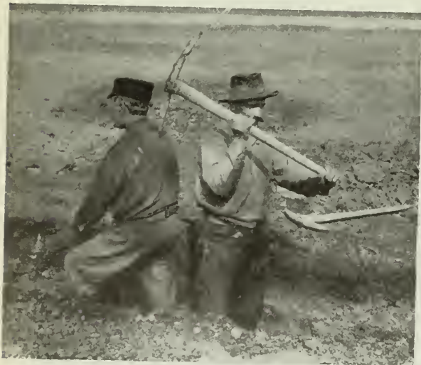
FIG. 27. EXCAVATION OR DITCHING, SHOWING LIABILITY TO SERIOUS ACCIDENT IF MEN WORK TOO CLOSE TOGETHER.
