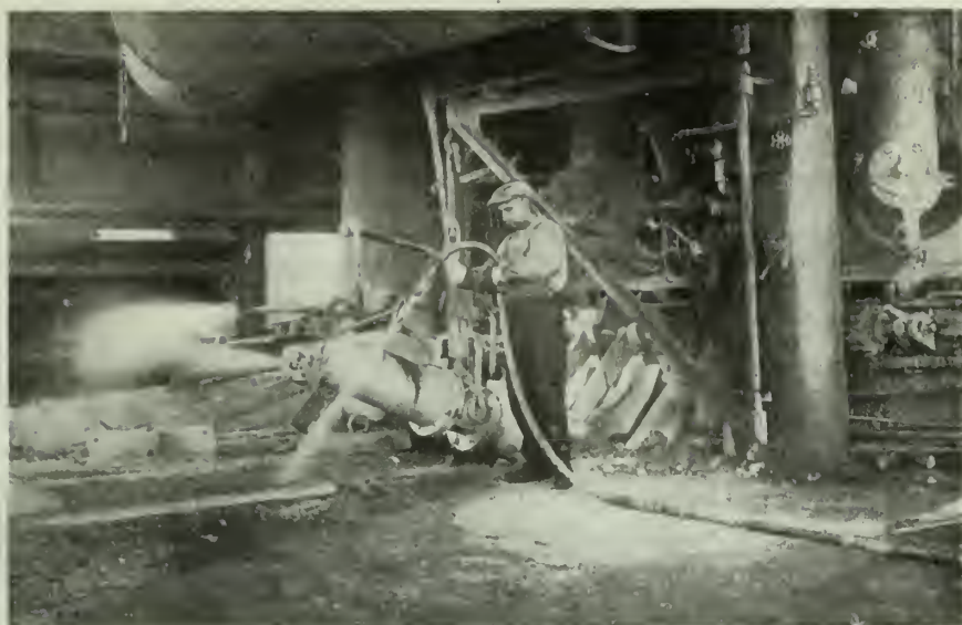
FIG. 19. UNSAFE WAY OF WETTING DOWN TROUGH AT "RID-UP." Short nozzle on the hose, man standing close to trough where he is exposed to an explosion of hot metal or steam.
