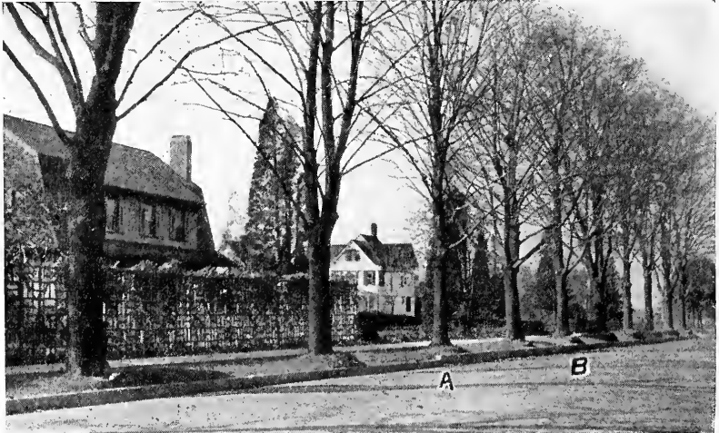
Fig. 23. Trees saved by mounding and raising curb when road was lowered. Note step in curb at A. Base of tree B is 30 inches above the gutter.
