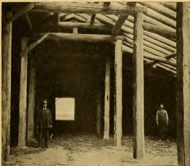
FIG. 112.—Interior view of same cellar showing roof construction and method of supporting it; also central driveway through the storage cellar. Messrs. Lou D. Sweet on the left and F. E. Sweet on the right.
