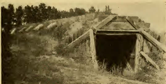
FIG. 115.—One of the cheaper types of partially sunken, earth-covered storage houses with earth retaining walls and side roof openings which may be used for filling the storage space or for ventilation. In the Greeley, Col., district.
