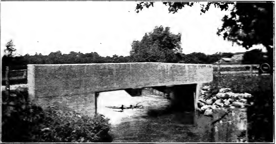
FIG. 111.—Parapet girder bridge (concrete). High class road. Span 25 ft. Width of roading 22 ft. Approximate cost (1920) $5000. Actual cost (1914) $2300.
