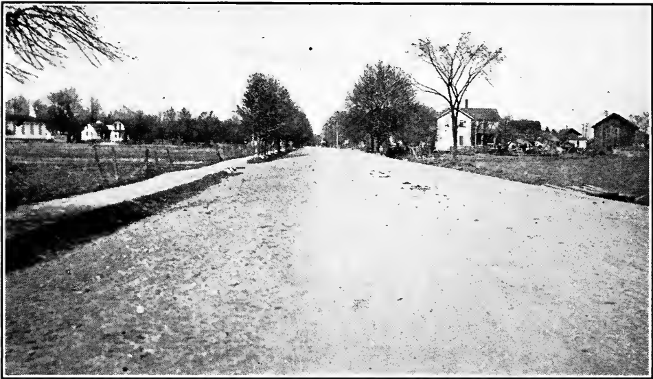
FIG. 5.—Typical penetration bituminous macadam (State Route No. 16 New York). Carries approximately 1500 vehicles per day. Note the easy shoulder slope which adds to the safety of traffic.
