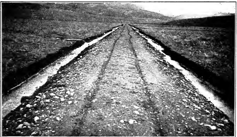
FIG. 78.—High turnpiking (gravelled) with deep ditches to raise road on flat above spring floods (Utah).
