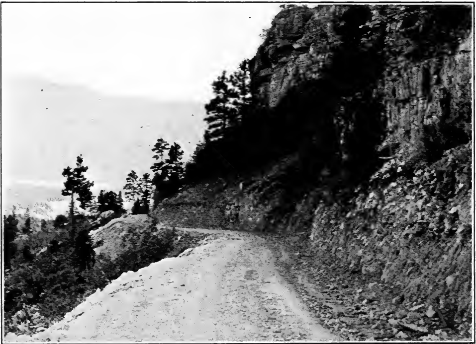
FIG. 8.—Typical unprotected mountain road. Illustrates the necessity for careful driving. Continuous guard rail would be prohibitive in cost except on a few of the main transcontinental routes.
