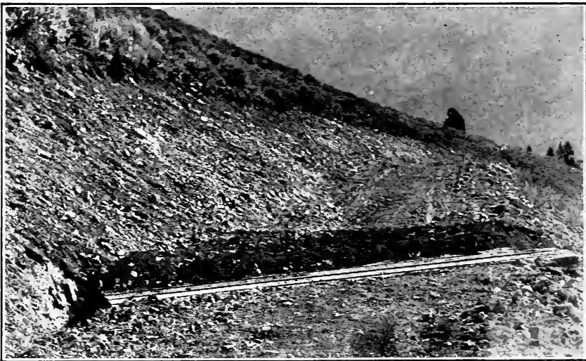
FIG. 97.—Open slat top relief culvert. Note angle with \text{C} of road. Pioneer road Colorado.
