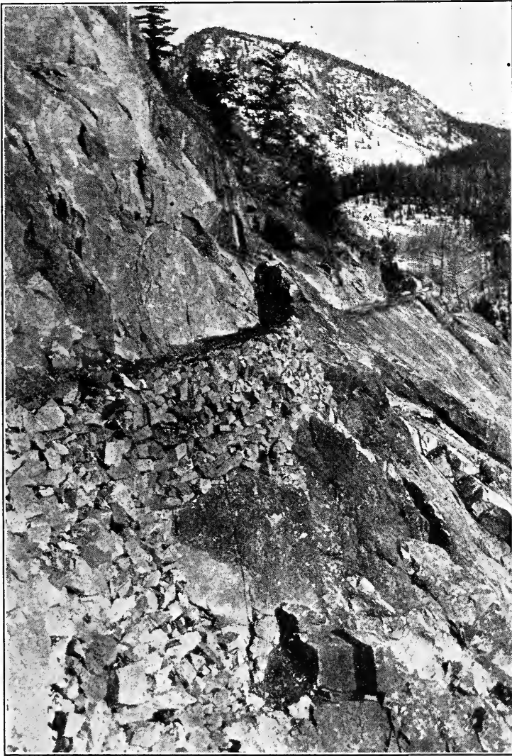
FIG. 83.—An example of poor unsafe wall construction.
