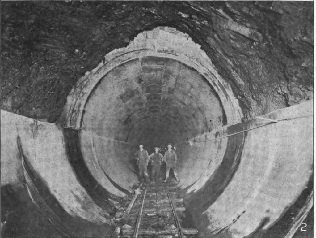
1 Catskill Aqueduct — Typical cut-and-cover aqueduct construction, showing excavated trench, steel forms, partial and complete concrete aqueduct and ungraded earth cover. The waterway is 17 feet high and 17½ feet wide, and has an area of 241 square feet
