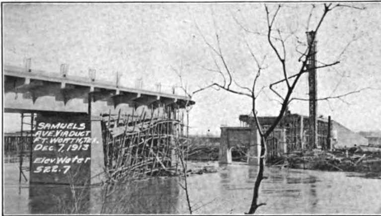
Courtesy of Mr. E. W. Robinson of the McKenzie Cons. Co., San Antonio, Texas. Fig. 475.—Samuels Avenue viaduct. View of wrecked river span falsework.
