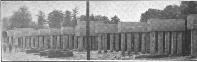
Courtesy of Mr. Maro Johnson, Engineer of Bridges and Buildings, I. C. R. R. FIG. 255.—Construction view of concrete pile trestle on Illinois Central R. R. near Obion, Tenn. Concrete bents ready for slabs.
