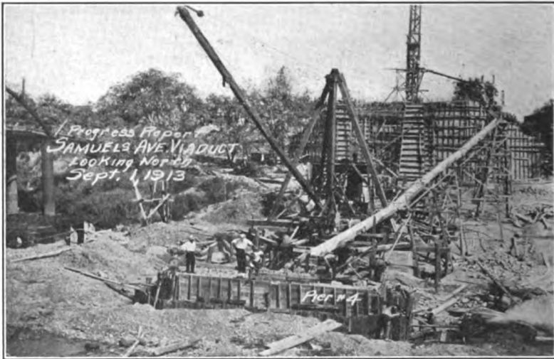
Courtesy of Mr. E. W. Robinson of the McKenzie Cons. Co., San Antonio, Texas. FIG. 467.—Samuels Avenue viaduct. Pulling pier forms with derrick, showing also spouting equipment for substructure work.
