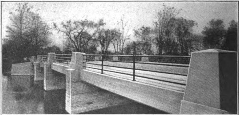
FIG. 398.—Flimsy gas-pipe rail compensated to some extent by heavy but awkward posts.
