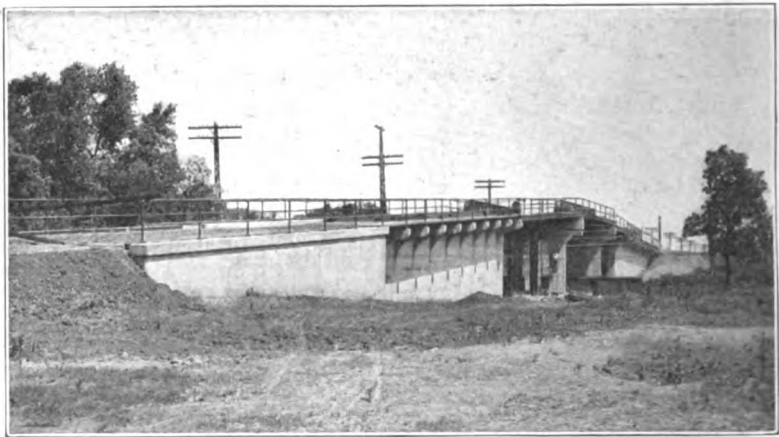
FIG. 371.—Lack of harmony due to combination of steel girders with concrete girders in the same structure.
