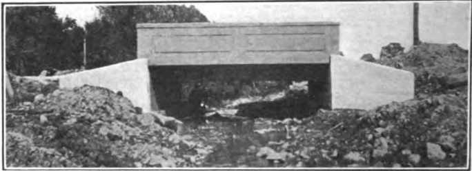
Courtesy of Mr. M. W. Torkelson, Bridge Engineer, Wisconsin Highway Commission. FIG. 247.—Christiana bridge over Brewery Creek, Town of Cross Plains, Dane County, Wis.
