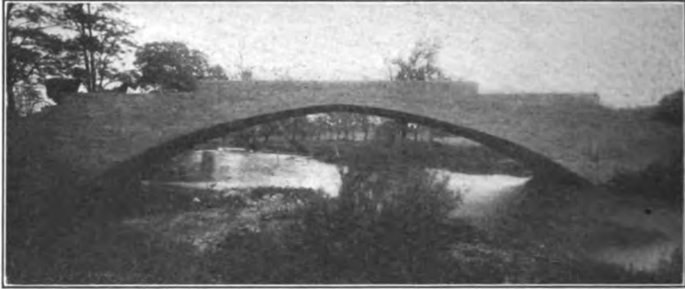
FIG. 393.—Unsightly arch in beautiful surroundings; no coping; no railing; unintentional break at crown due to careless erection.
