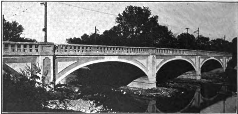
FIG. 391.—Undesirable effect of triangular panels in retaining walls at each end of bridge. Raised panels on arches objectionable. Form of panels inartistic, particularly the feature that maintains a uniform thickness of arch ring. The bridge has no camber, resulting in appearance of sag at crowns. Plinth and cap of railing inadequate.
