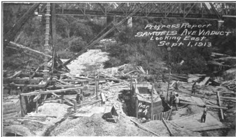
Courtesy of Mr. E. W. Robinson of the McKenzie Cons. Co., San Antonio Texas. FIG. 468.—Samuels Avenue viaduct. Pulling cofferdam sheeting with derrick.
