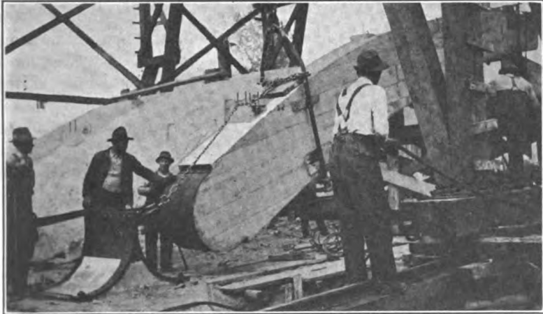
Courtesy of Mr. Wm. M. Thomas, Consulting Engineer, Los Angeles, Cal.
