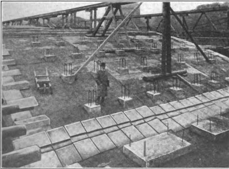
FIG. 517.—Rudolfinum bridge at Prague. View showing skewback-hinge blocks and spandrel column bases. (Note that the intermediate concrete columns have concrete bases and the exterior cut-stone face columns have cut-stone or voussoir bases. Also note round timber framework.)
