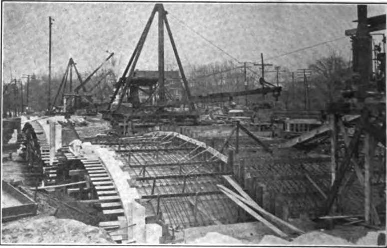
Courtesy of Mr. Charles W. Cole, City Engineer, Mishawaka, Ind. FIG. 88. —Construction view of North Michigan Street bridge, South Bend, Indiana.
