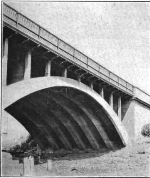
FIG. 10E.—Wealthy Street bridge, Grand Rapids, Mich. Note thin slab between arch ribs at extrados.
