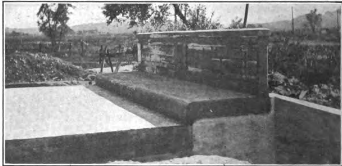
Courtesy of Mr. M. W. Torkelson, Bridge Engineer, Wisconsin Highway Commission. FIG. 248.—Construction view of Christiania bridge, Town of Cross Plains, Dane County, Wis.
