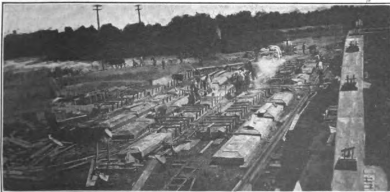
Courtesy of Mr. Wm. M. Thomas, Consulting Engineer, Los Angeles, Cal.
