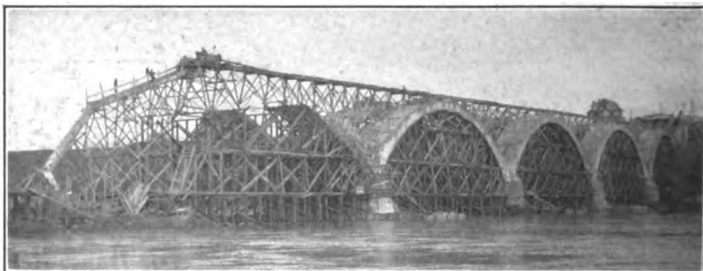
Courtesy of Mr. Daniel B. Luten, Consulting Engineer, Indianapolis. FIG. 97.—Construction view of bridge over Saskatchewan River at Saskatoon, Canada.
