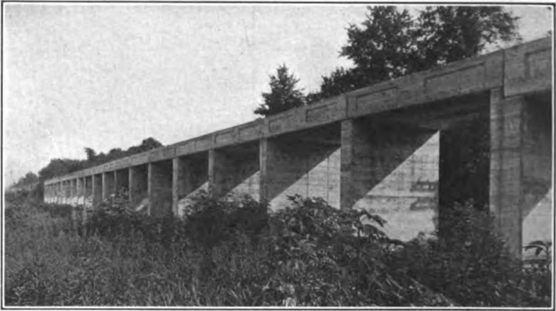
Courtesy of Mr. Maro Johnson, Engineer of Bridges and Buildings, I. C. R. R. FIG. 260.—Solid benchwall type of concrete trestle on Illinois Central R. R. near New Athens, Ill.
