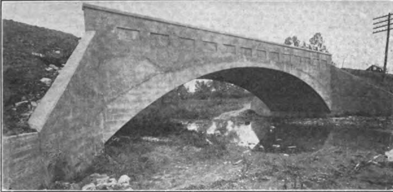
FIG. 395.—Lack of coping and plinth ruins an otherwise acceptable structure. Improper location of panels accentuates absence of coping. Un-sightly discoloration on spandrel face due to improper selection of construction joints.
