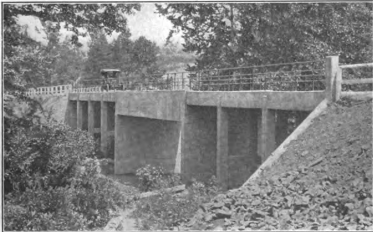
FIG. 381.—Poorly-designed girder bridge. Unequal spans are not easily harmonized. Inadequate supports; flimsy railing.
