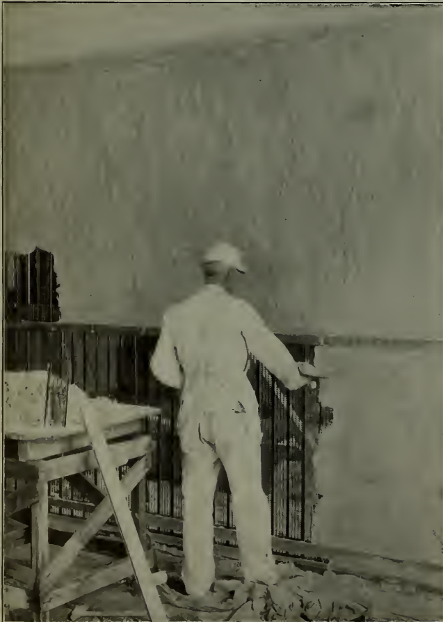
Hy-Rib Partition, Trussed Concrete Building, Detroit, Mich. Note grounds for base-board and chair-rail.
