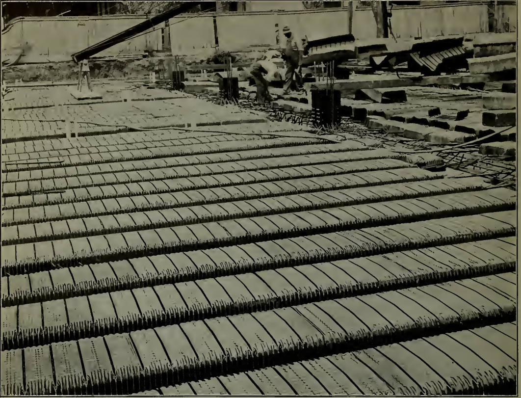
Use of Floretyles at Couzens Building, Detroit, Mich. Note the true lines of joists and the great rigidity of Floretyles.
