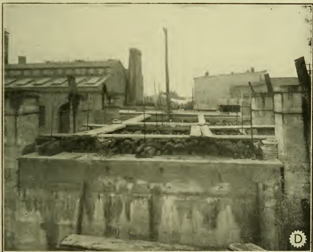
A uniform load of 150 to 160 pounds per square foot was laid on top of the du Mazuel construction, and steel level rods were placed thereon for determining deflections.
