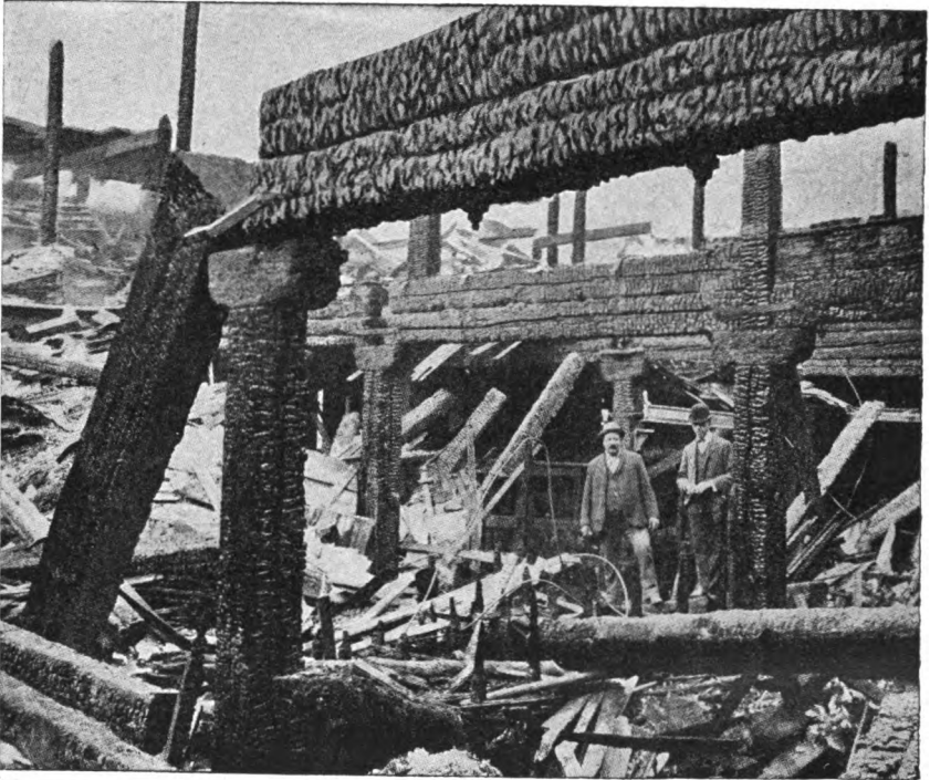
Fig. 14. What Is Left of a "Slow-Burning", "Mill-Constructed" Building after a Fire
