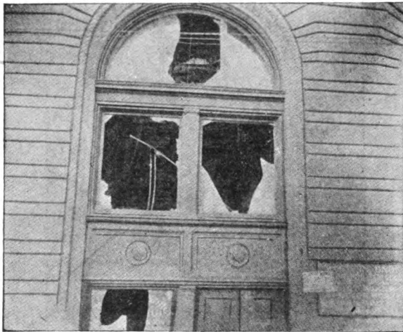
Fig. 23. The Inadequacy of Ordinary Glass Fire went through these windows as it would through paper.
