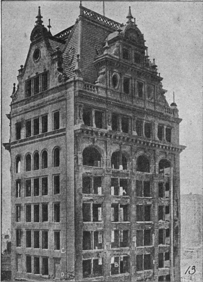
Fig. 38. Note Effect of a Fire Upon the Stone Work of the Upper Parts of a Tall Building
