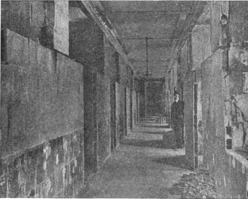
Fig. 3. Wooden Sash in Tile Partitions This construction permits fire to travel from room to room
