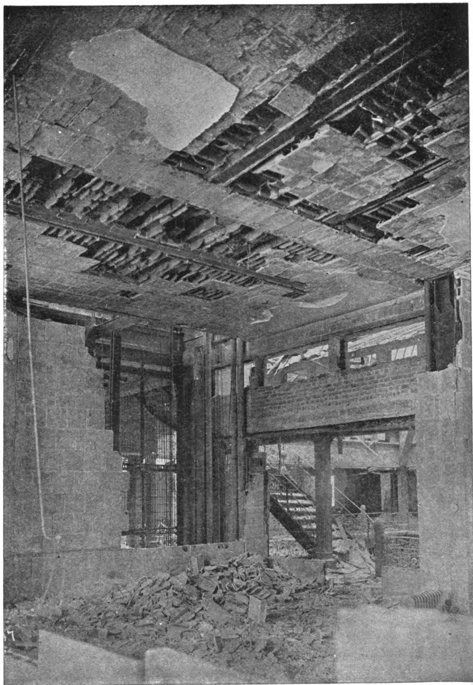
Fig. 26. The Effect of Fire Upon Too Thin and Dense Hollow Tile
