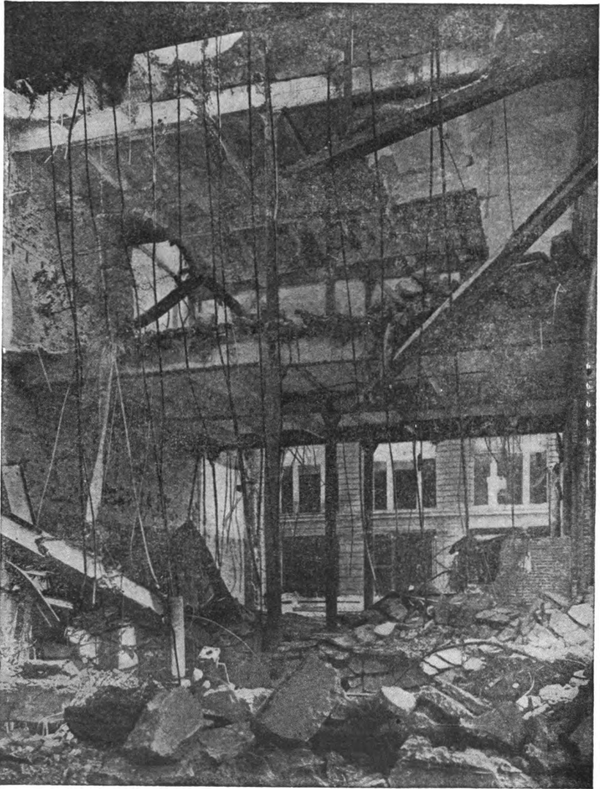
Fig. 9. Fire's Effect Upon a Building of Cast-Iron Columns, Steel Girders, Concrete Beams and Concrete Slab Floors
