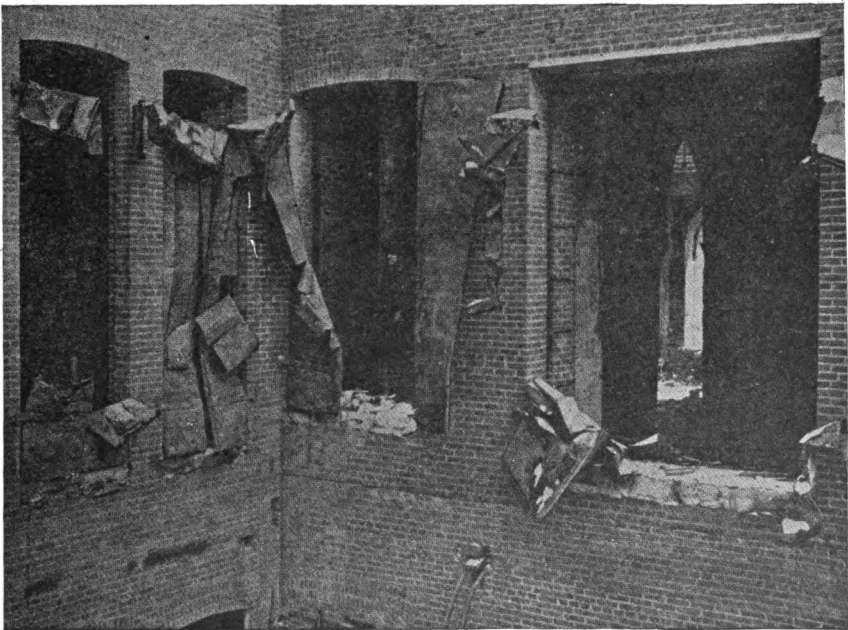
Fig. 18 Ineffective Fire Shutter Protection
