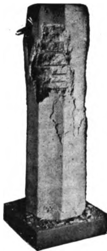
FIG. 73.—Spalling of the outer concrete shell.
