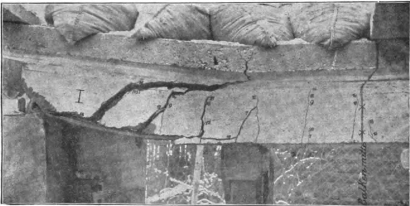
FIG. 119.—Failure cracks in the vicinity of the points of support of a concrete T-beam reinforced with only straight round rods.
