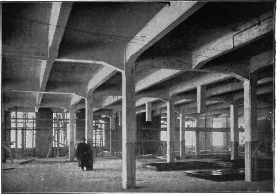
FIG. 208.—Hanging columns for the carrying of shafting in the Speyer cotton mill on the Rhine.
