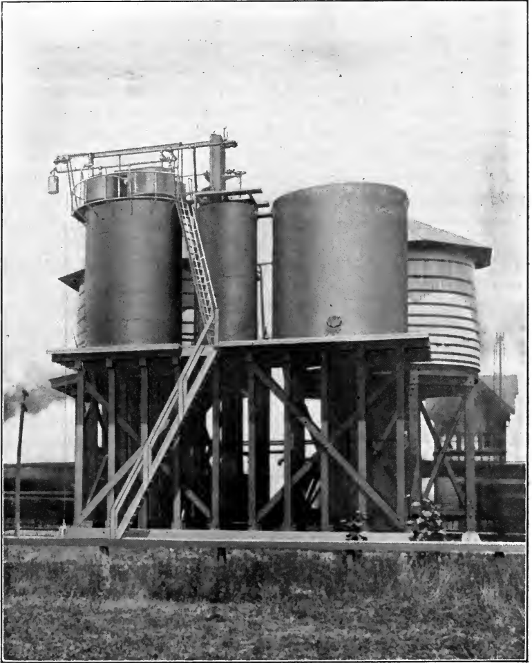
FIG. 47.—Water-softening Plant, Middlepoint, Ohio—Pennsylvania Lines West of Pittsburgh.
